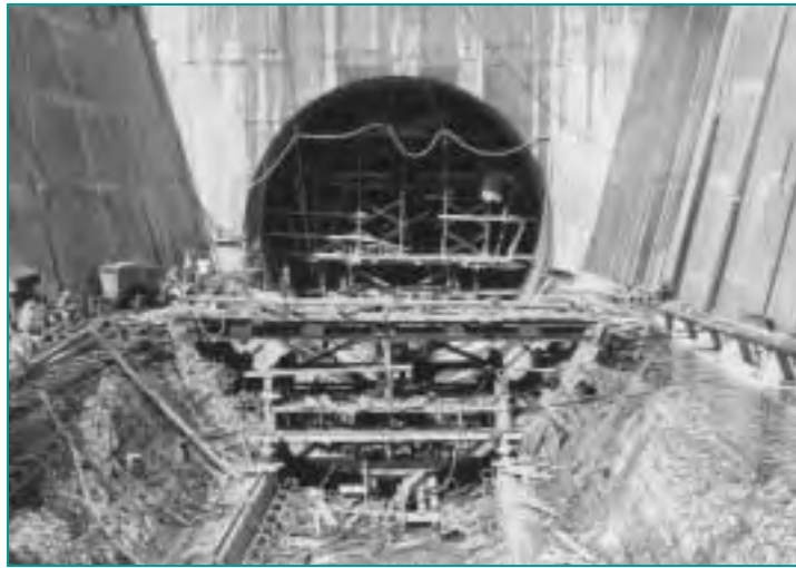
Mica Dam, shown here under construction, is one of three Canadian projects that are among the most recent major projects built on the river system. They have greatly increased the ability to control streamflows.
