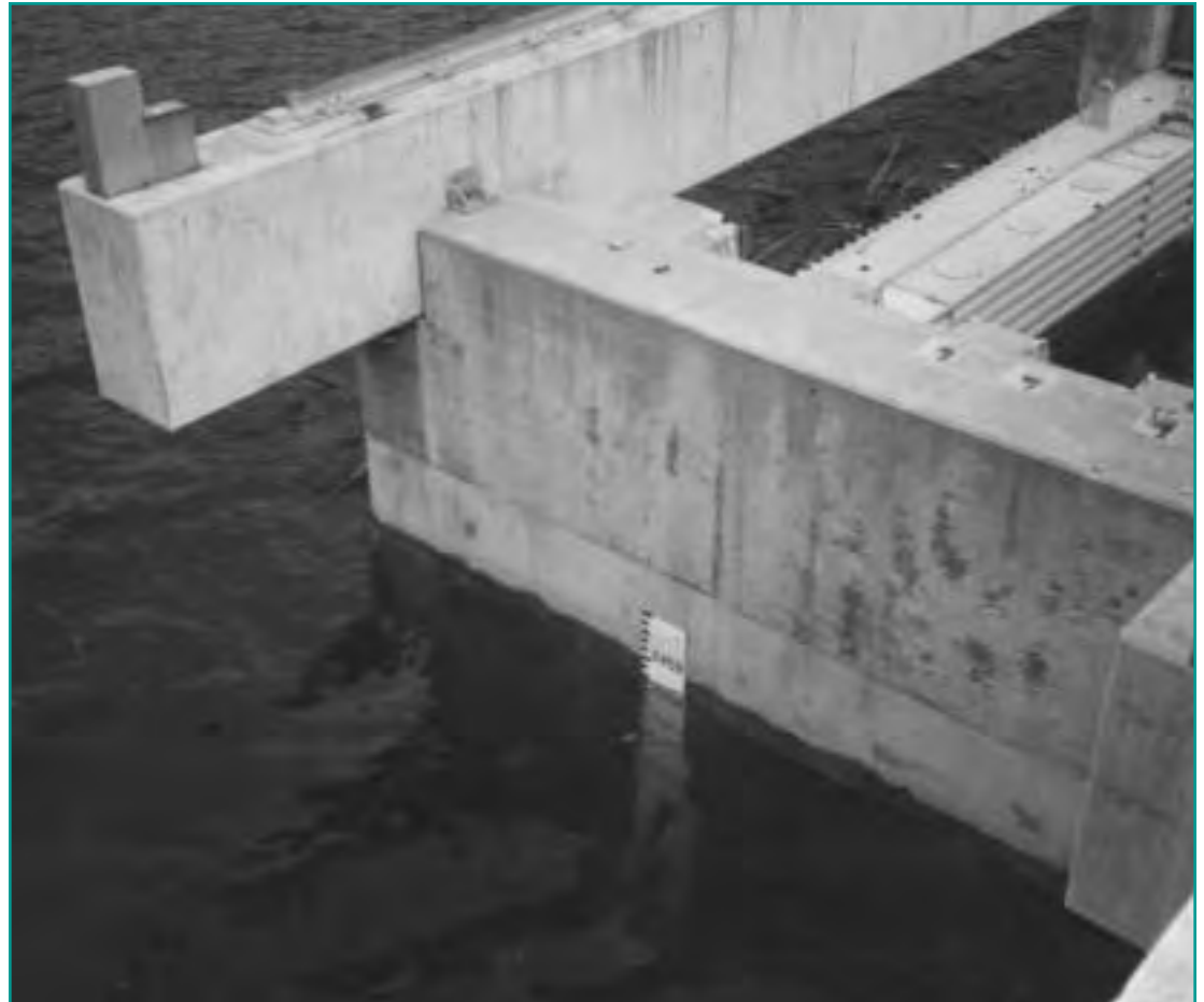
Indicators, like this one at Libby Dam, are used to gauge the water level at each reservoir. Efforts are made to refill the reservoirs every year. Runoff is usually adequate to refill reservoirs about three out of every four years.
