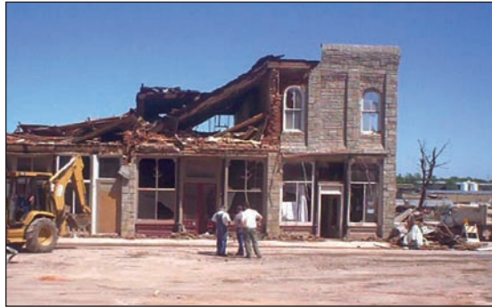
Surveying the damage in Stockton, Mo.
