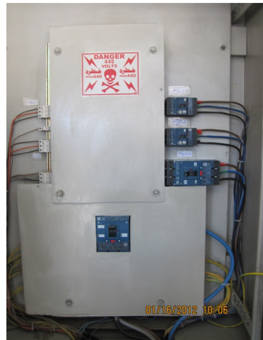
Main electrical panel at Police District 3 in Kabul, SIGAR site inspection, January 2012.
