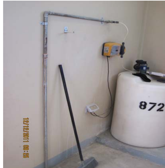
Figure 8 - Corroded Steel Pipe at the Joint Regional Afghanistan Security Forces Compound Water Treatment System
