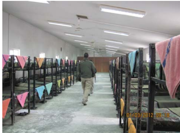
Figure 5 - Lights and Fans Operational in Barracks at Camp Shaheen in Mazar-e Sharif, Balkh
