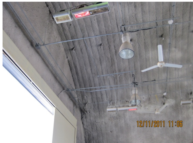
Figure 7 - Disconnected Heating Units in 8 th Commando Camp Maintenance Building
