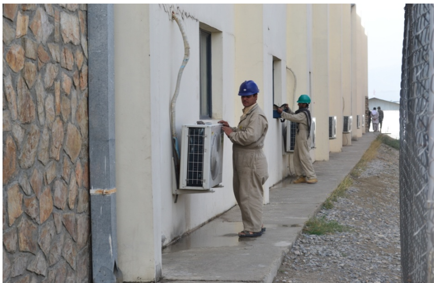
O&M trainees repairing heating and air conditioning units of barracks at the Kabul Military Training Center, SIGAR site inspection, October 2011.
