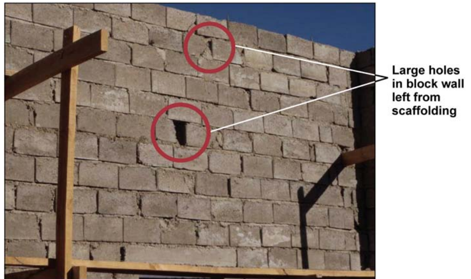
Figure 4: Cement Block Wall with Large Holes That Remained When Scaffolding Was Removed
