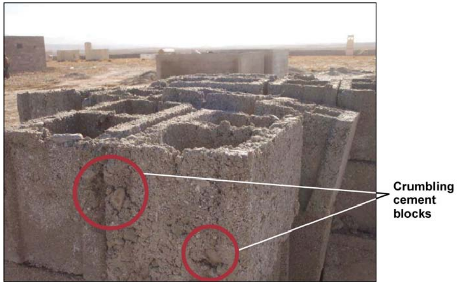
Figure 2: Poor-Quality Materials—Crumbling Cement Blocks
