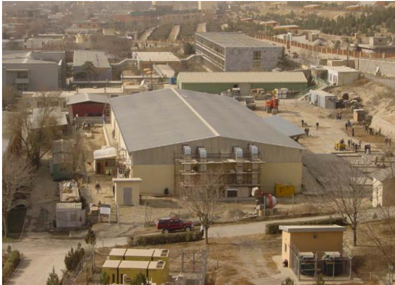
A new Class VIII Inventory Warehouse under construction near the National Military Hospital, Kabul Afghanistan, December 6, 2010. The existing Class VIII warehouse is the green building to the rear. The existing warehouse was poorly lit, not well organized, and did not have “on-hand” pharmaceutical inventory arranged by location.
