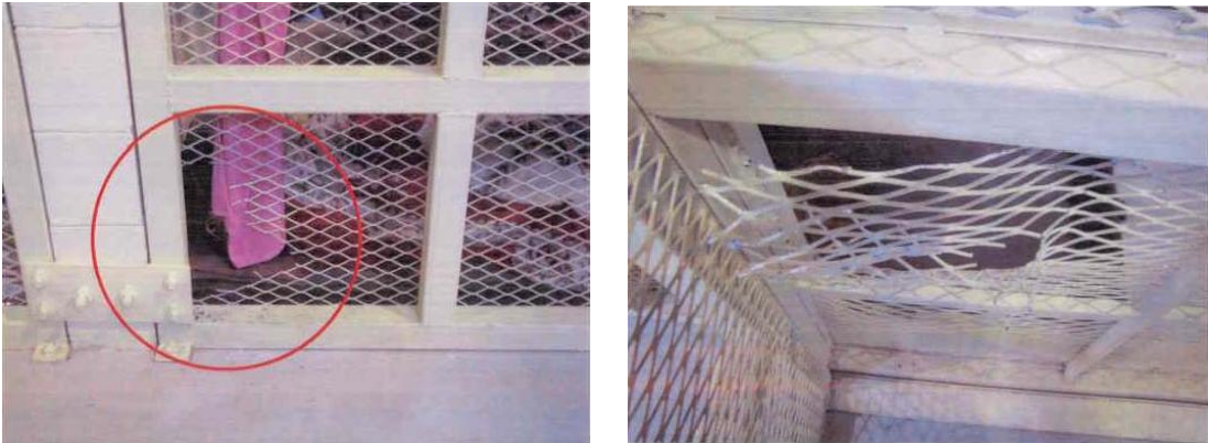
Figure 2. Examples of Cell Damage
