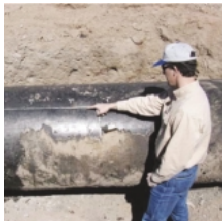
A Pacific Gas & Electric worker points to one of the discovered leaks in the exposed pipe.
