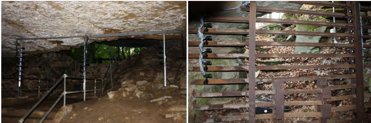
Figure 1. The GateKeeper beam-break system installed on independent uprights at Wyandotte Cave, Crawford County, IN, (left) and on the gate at James Cave, Edmonson County, KY, (right). Both views are from inside the caves.
