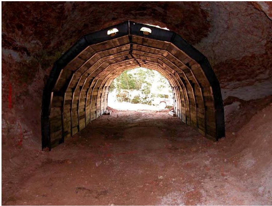
Figure 2. Steel arch with wooded cross beam system in an abandoned mine in Southern Illinois.
