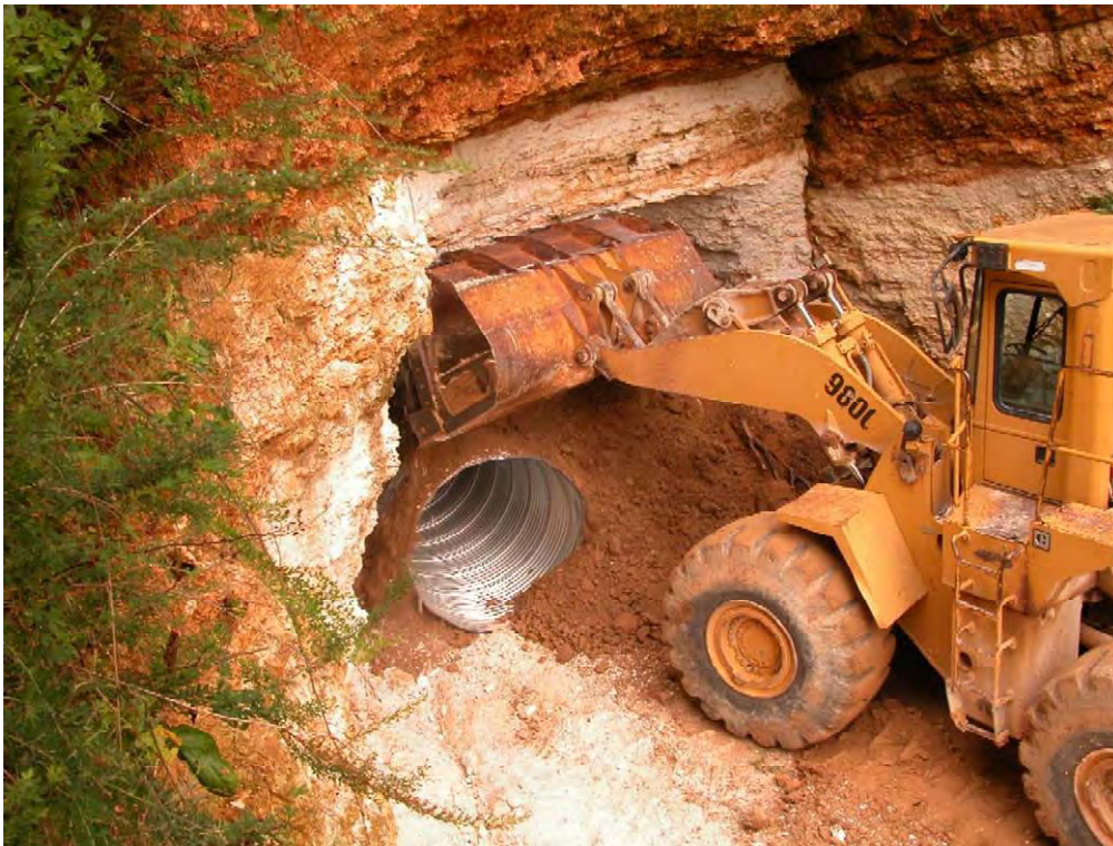
Figure 7. Closure of lower entrance in Birk 2 mine to reducing air flow for better control of internal mine temperature.
