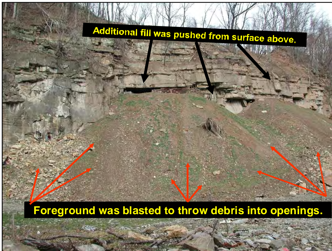
Figure 2. Existing large tunnels on state land needed to be closed for safety reasons. Fill was blasted and pushed into 3 openings. Two gated openings at the top provided an exchange of air and allowed cold air to drop into the lower portions of the mine. The next winter, Indiana bats were found in the site for the first time.
