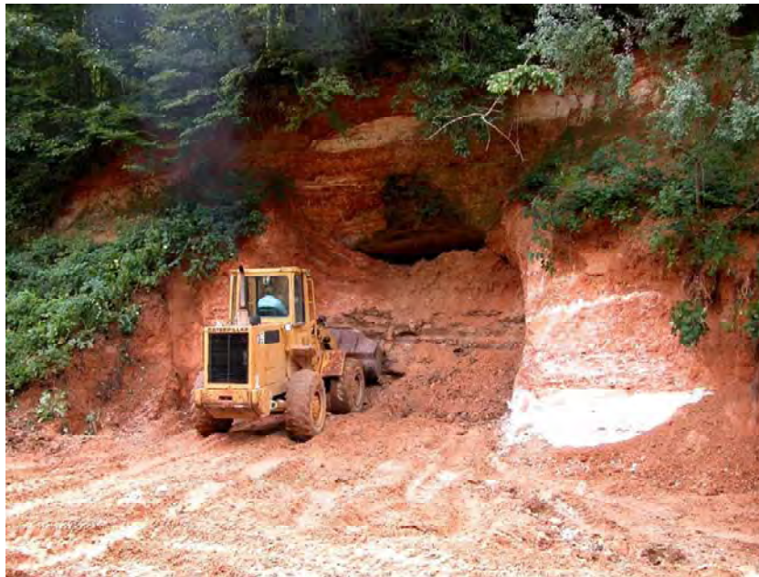
Figure 1. Unstable mine entrance being excavated in Southern Illinois.
