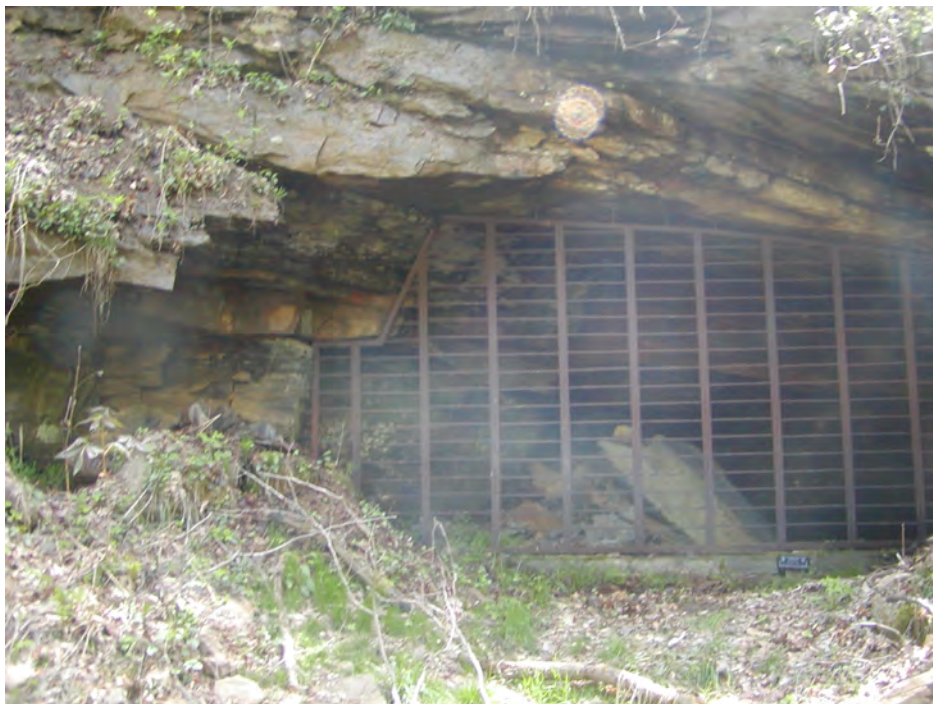
Figure 3. Bat gates installed to protect bat roosting and hibernacula in portal 2D.
