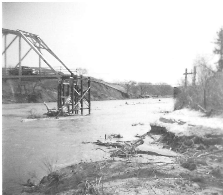
Niobrara River near Verdel, Nebr. Flood of March 27, 1960, washed out the right (south) section of bridge. (Photograph by J. A. Anderson, U.S. Geological Survey)
