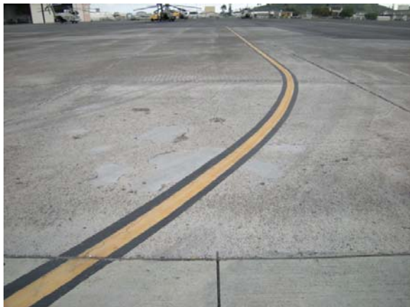
Figure 3-19: Damaged Area "d," pitted and repaired area in the center of the photo. Photo taken looking north, toward Hangar 1.
