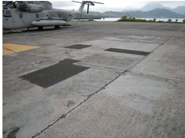
Figure 3-22: Damaged Area "e." Photo taken looking south, toward the bay.
