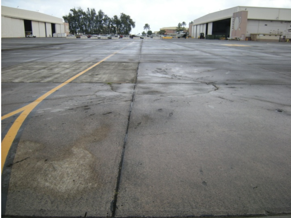
Figure 3-29: Bomb Crater "2," Large repair in the center of the photo; radial damage surrounding the repair; replaced concrete section in the center left of the photo. Photo taken looking northeast, between Hangars 2 & 3.
