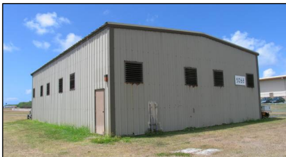
Figure 3-10: Facility 5068 is a baloncarbon reclamation facility constructed in 1991. Photo taken in August 2009.
