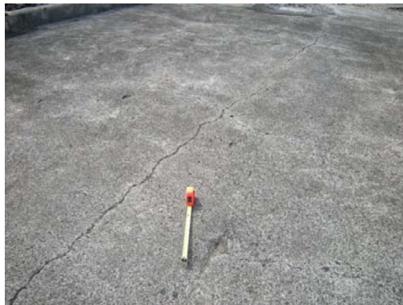
Figure 28: Damaged Area "k," apparent bullet impact mark in Seaplane Ramp 3. Photo taken looking south, toward the bay.
