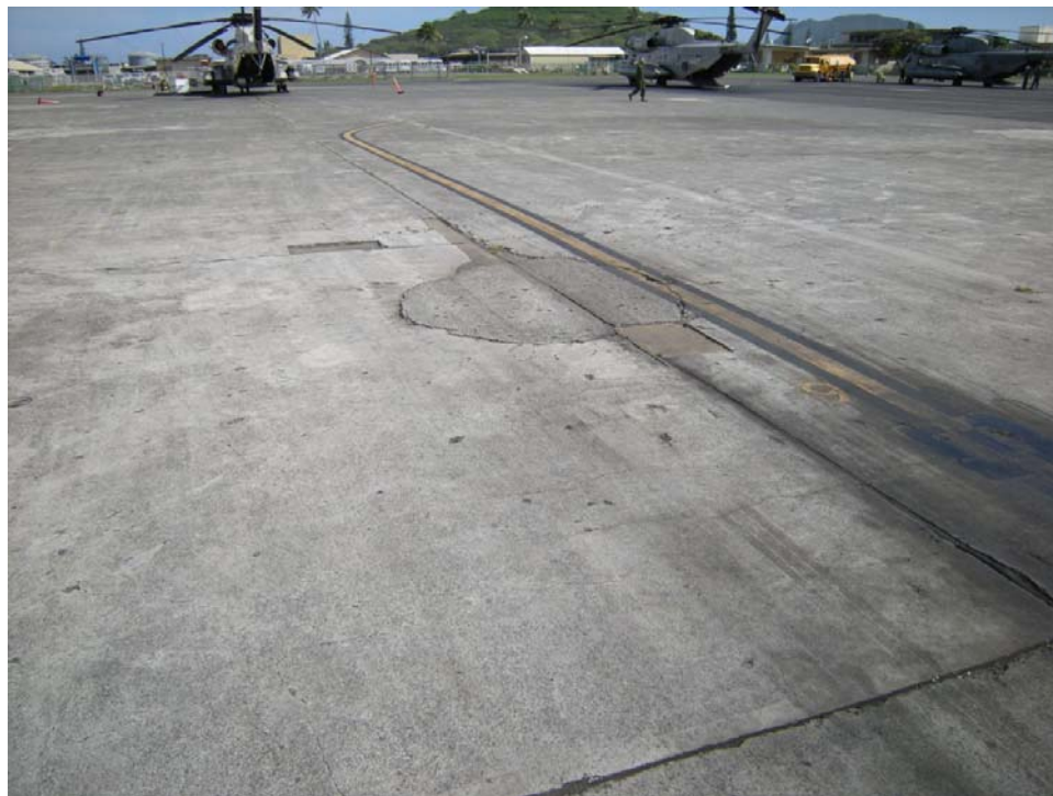
Figure 3-12: Bomb Crater "1" in the center of the photo. Photo taken looking southeast.
