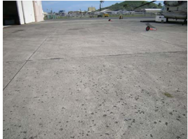
Figure 3-14: Damaged Area "a." Photo taken looking northwest.
