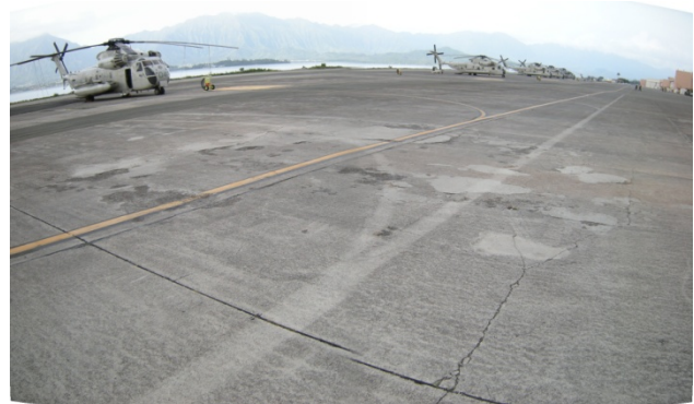
Figure 3-24: Damaged Area "f." Photo taken looking west, toward the bay.
