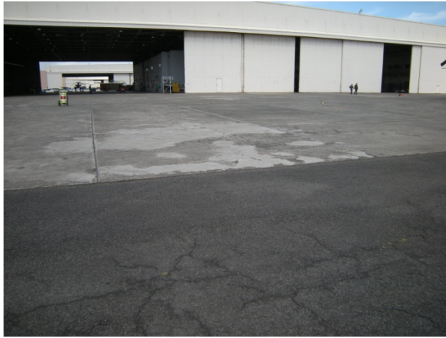
Figure 3-17: Damaged Area "c," the repaired concrete area in the center of the photo. Photo taken looking toward Hangar 1.
