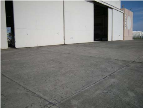
Figure 3-13: Damaged Area "a." Photo taken looking north, toward Hangar 1.
