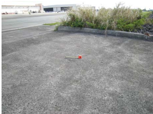
Figure 27: Damaged Area "k," apparent bullet impact mark in Seaplane Ramp 3. Photo taken looking east, toward Hangars 1 & 2.
