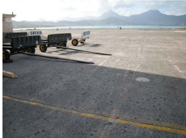
Figure 24: Damaged Area "i." Photo taken looking southwest, toward the bay.
