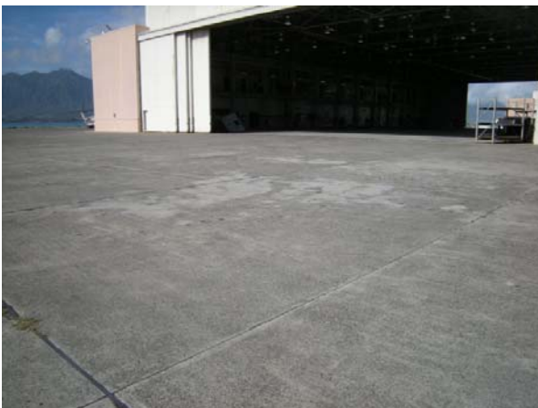
Figure 3-15: Damaged Area "b." Photo taken looking west, toward Hangar 1.
