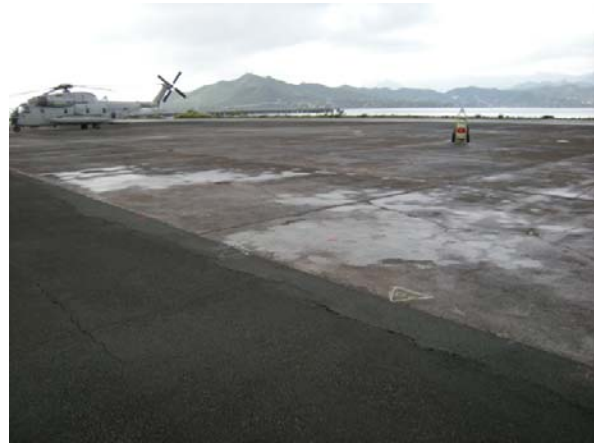
Figure 3-26: Damaged Area "g." Photo taken looking south.
