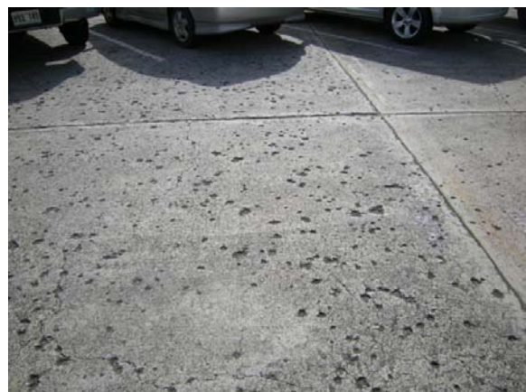
Figure 3-28: Damaged Area "h." Photo taken looking northeast.
