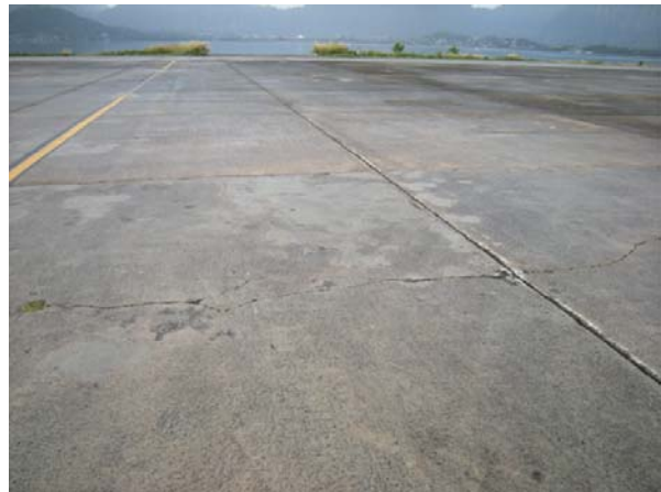
Figure 26: Damaged Area "j." Photo taken looking southeast, toward the bay.
