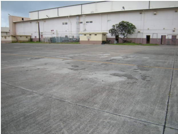
Figure 3-23: Damaged Area "f," pitted and repaired area in the center of the photo. Photo taken looking north, toward Hangar 1.
