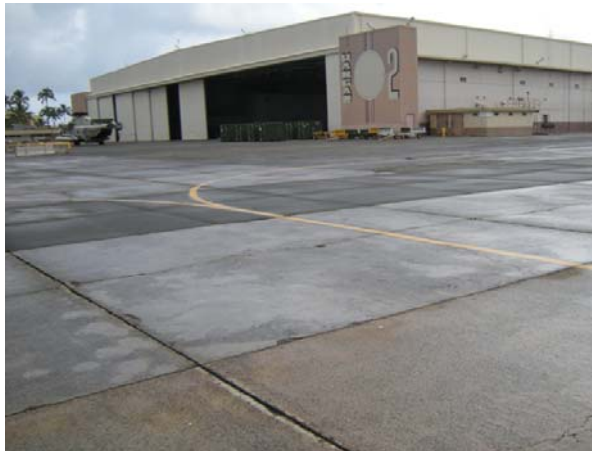
Figure 25: Damaged Area "j," pitted and repaired areas in the center and lower left of the photo. Photo taken looking east, toward Hangar 2.
