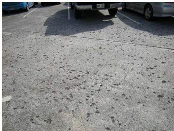
Figure 3-27: Damaged Area "h." Photo taken looking northeast.
