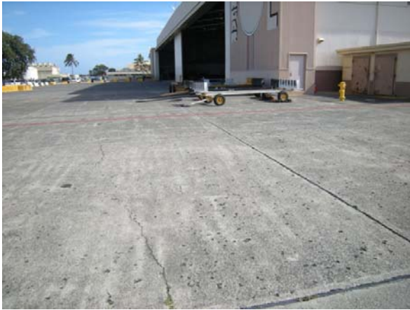
Figure 23: Damaged Area "i." Photo taken looking northeast, toward Hangar 2.
