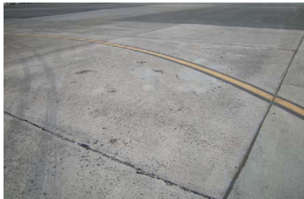
Figure 3-20: Damaged Area "d." Photo taken looking west.
