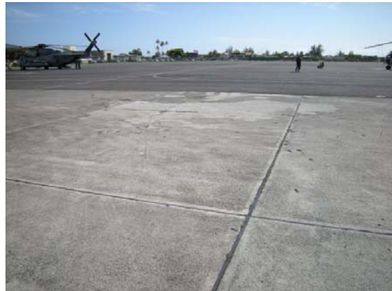
Figure 3-18: Damaged Area "c." Photo taken looking east.
