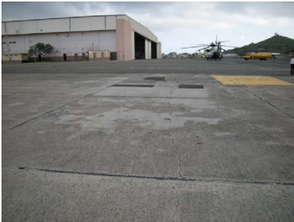
Figure 3-21: Damaged Area "e," pitted and repaired area in the center of the photo. Photo taken looking northeast, toward Hangar 1.
