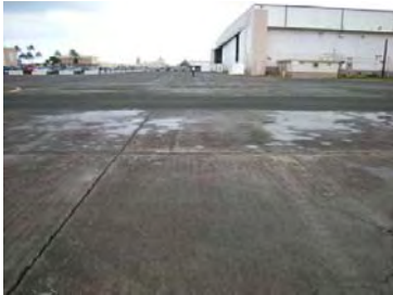
Figure 3-25: Damaged Area "g." Photo taken looking northeast, toward Hangar 1.
