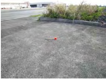
Figure 27: Damaged Area "k," apparent bullet impact mark in Seaplane Ramp 3. Photo taken looking east, toward Hangars 1 & 2.
