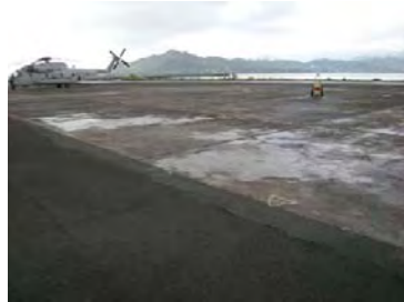
Figure 3-26: Damaged Area "g." Photo taken looking south.
