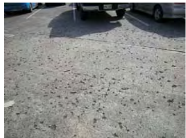
Figure 3-27: Damaged Area "h." Photo taken looking northeast.
