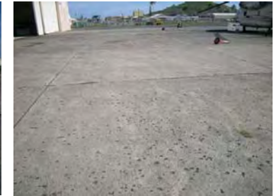
Figure 3-14: Damaged Area "a." Photo taken looking northwest.
