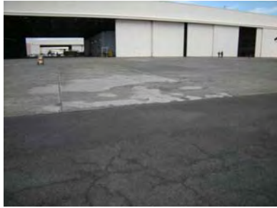
Figure 3-17: Damaged Area "c," the repaired concrete area in the center of the photo. Photo taken looking toward Hangar 1.
