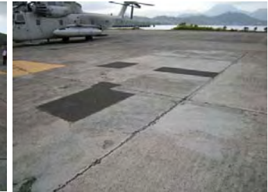
Figure 3-22: Damaged Area "e." Photo taken looking south, toward the bay.
