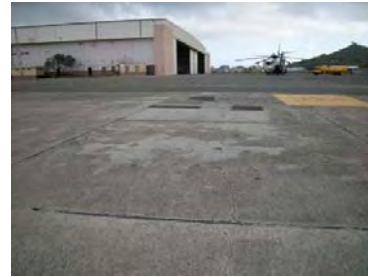
Figure 3-21: Damaged Area "e," pitted and repaired area in the center of the photo. Photo taken looking northeast, toward Hangar 1.
