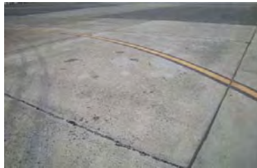
Figure 3-20: Damaged Area "d." Photo taken looking west.
