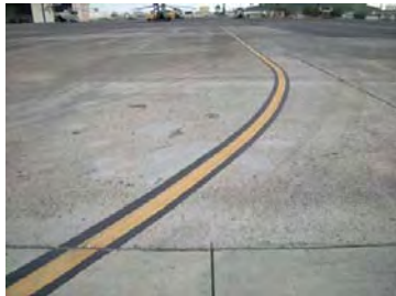
Figure 3-19: Damaged Area "d," pitted and repaired area in the center of the photo. Photo taken looking north, toward Hangar 1.
