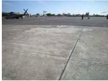
Figure 3-18: Damaged Area "c." Photo taken looking east.
