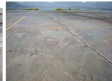
Figure 26: Damaged Area "j." Photo taken looking southeast, toward the bay.
