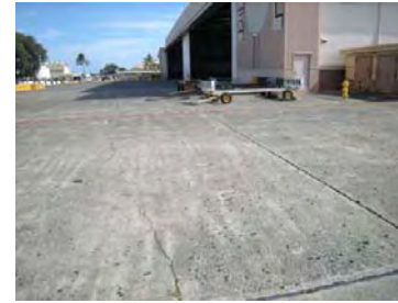
Figure 23: Damaged Area "i." Photo taken looking northeast, toward Hangar 2.
