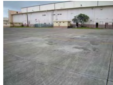
Figure 3-23: Damaged Area "f," pitted and repaired area in the center of the photo. Photo taken looking north, toward Hangar 1.
