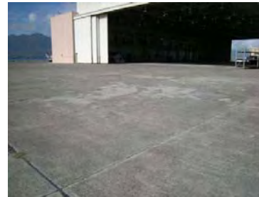
Figure 3-15: Damaged Area "b." Photo taken looking west, toward Hangar 1.
