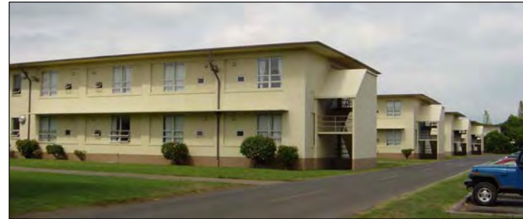
Figure 6-3: Enlisted Men's Barracks from May 2004. Note the added aluminum-sash windows which do not fill the window openings
