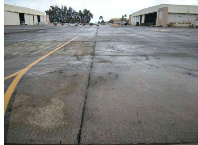
Figure 3-29: Bomb Crater "2." Large repair in the center of the photo; radial damage surrounding the repair; replaced concrete section in the center left of the photo. Photo taken looking northeast, between Hangars 2 & 3.
