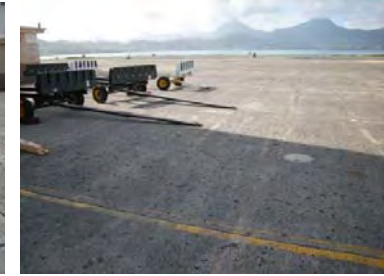
Figure 24: Damaged Area "i." Photo taken looking southwest, toward the bay.
