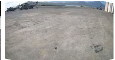
Figure 3-16: Damaged Area "b." Photo taken looking southwest.
