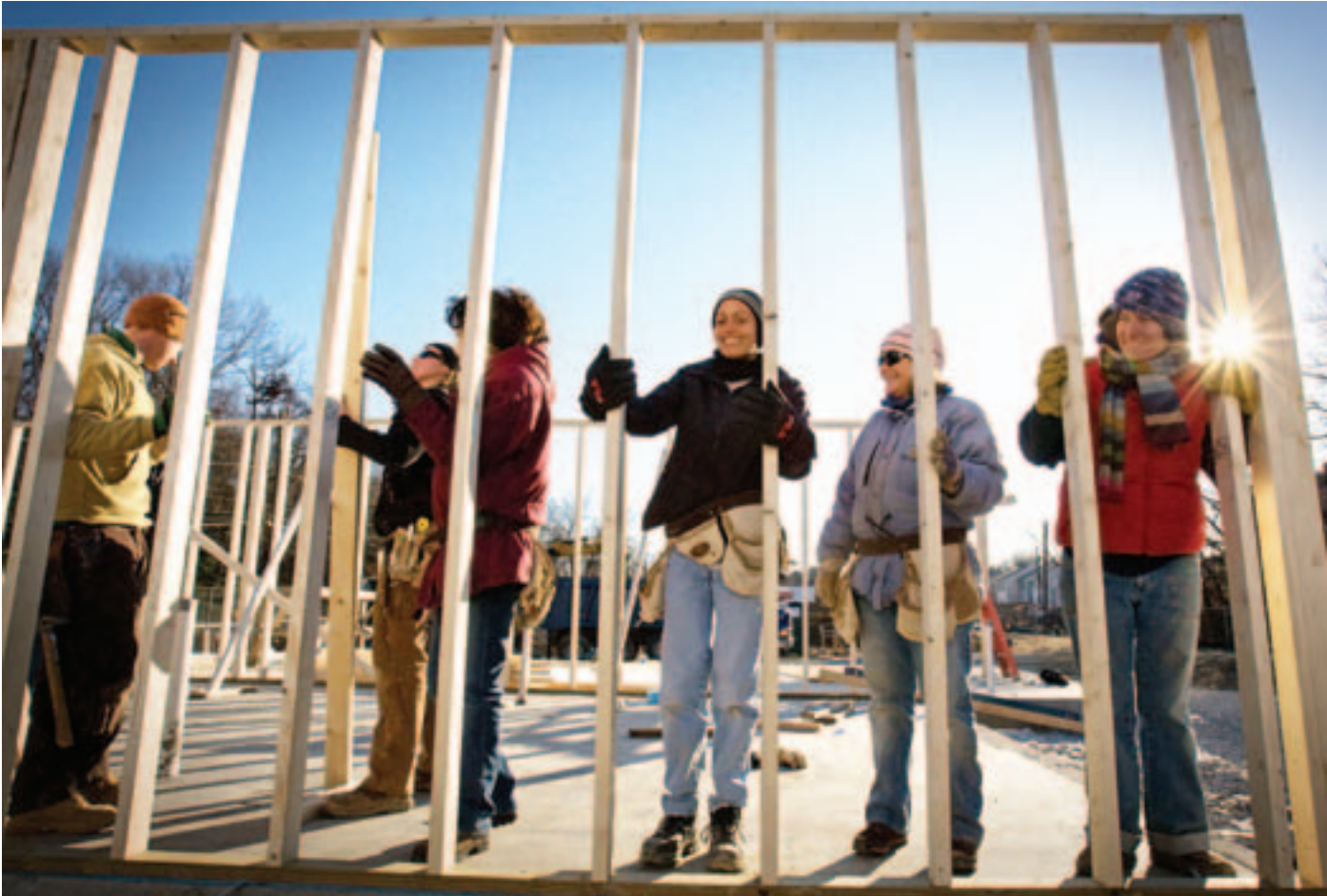
AmeriCorps members work with volunteers from Habitat for Humanity to build a house on the Martin Luther King, Jr. Day of Service.
