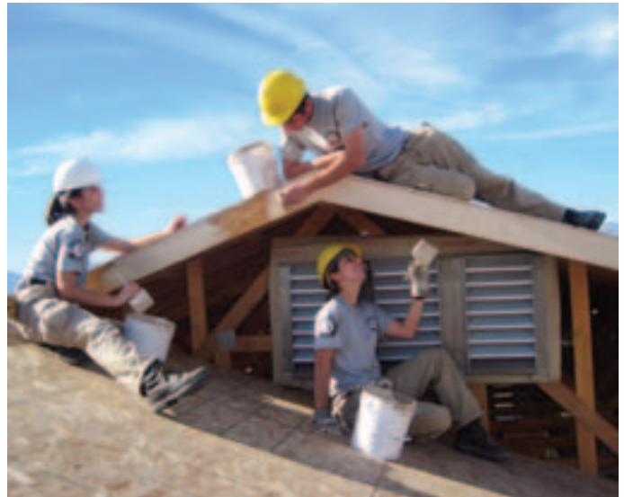
AmeriCorps NCCC members rebuild a house in the wake of Hurricane Katrina.
