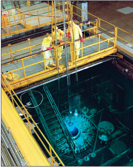
Technicians replace a fuel element at the High-Flux Isotope Reactor at Oak Ridge National Laboratory.
