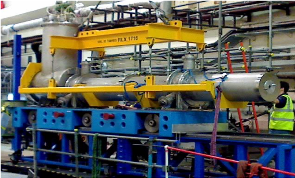
Figure 6: Photo of Decay Solenoid prior to its installation into the ISIS-vault shielding wall.
