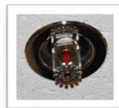
Sprinkler systems use bismuth, indium, and tin to trigger discharge of water to suppress fires.
