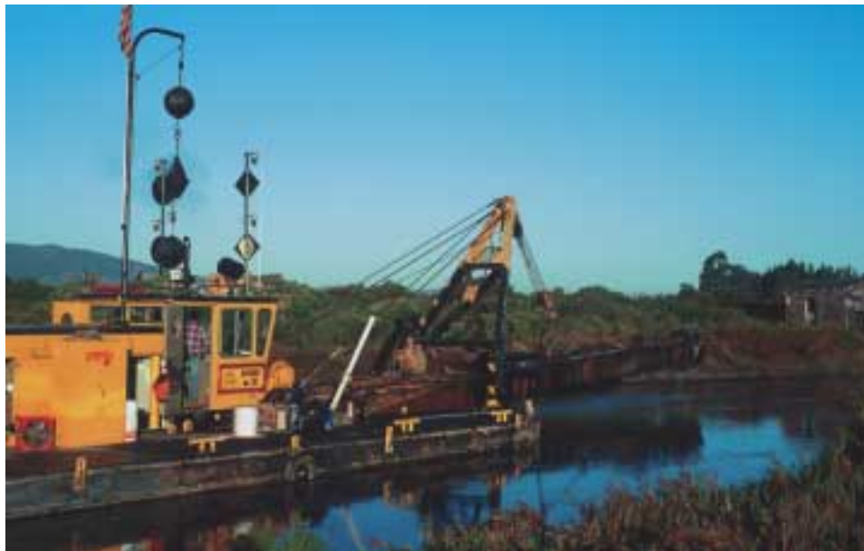
Dredge work was done both to enlarge channels, thereby restoring tidal action in Tolay Creek, and to improve levees to protect adjacent farmland.
