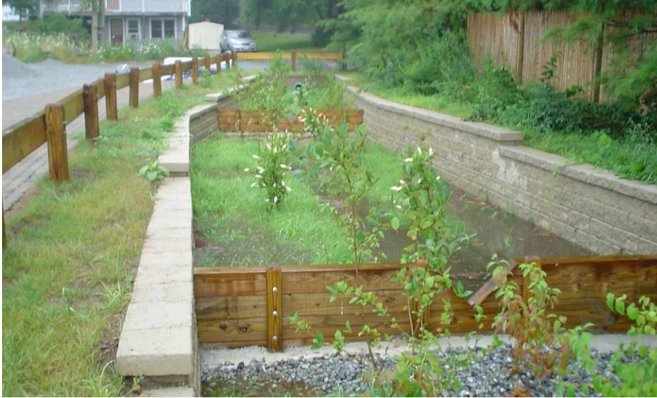
Figure 5-27. Roadside swale with wood check dams.
