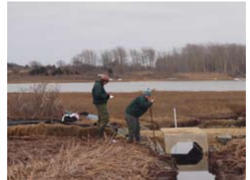
Culvert being restored at Medouie Creek to improve tidal flow. Photo credit: NOAA
