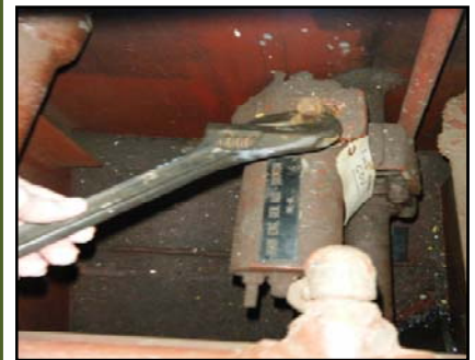
Figure 2: Valve fitting makes it difficult to determine if the valve is open or closed.
