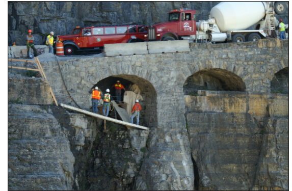
As construction continues, the Going-to-the-Sun Road remains open to nearly 500,000 vehicles each year.
