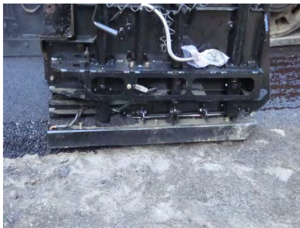
Figure 53. Side view of Carlson end gate.
