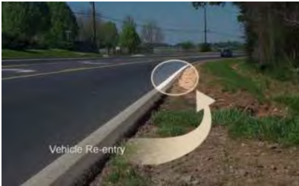
Figure 5. Vertical drop off at pavement edge. (FHWA Safety Edge SM PowerPoint)
