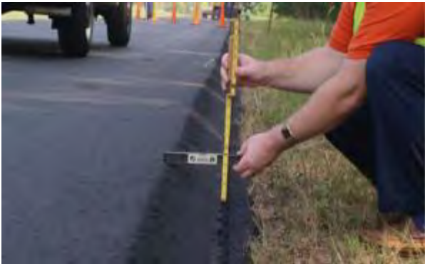
Figure 6. Sloping edge produced by pavement edge hardware. (FHWA Safety Edge SM PowerPoint)
