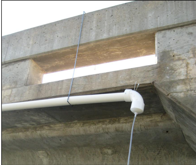
Figure 2.5 Bridge gutter installed at Highway 64 over the Platte River near Leshara, NE
