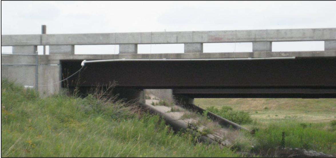
Figure 2.7 Bridge gutter installed at I-80 over Little Salt Creek site near 27 th Street exit in Lincoln, NE
