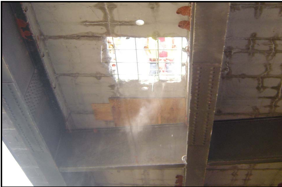
Figure 3.18 – Turner Turnpike Bridge 14.4 Deck Failure
