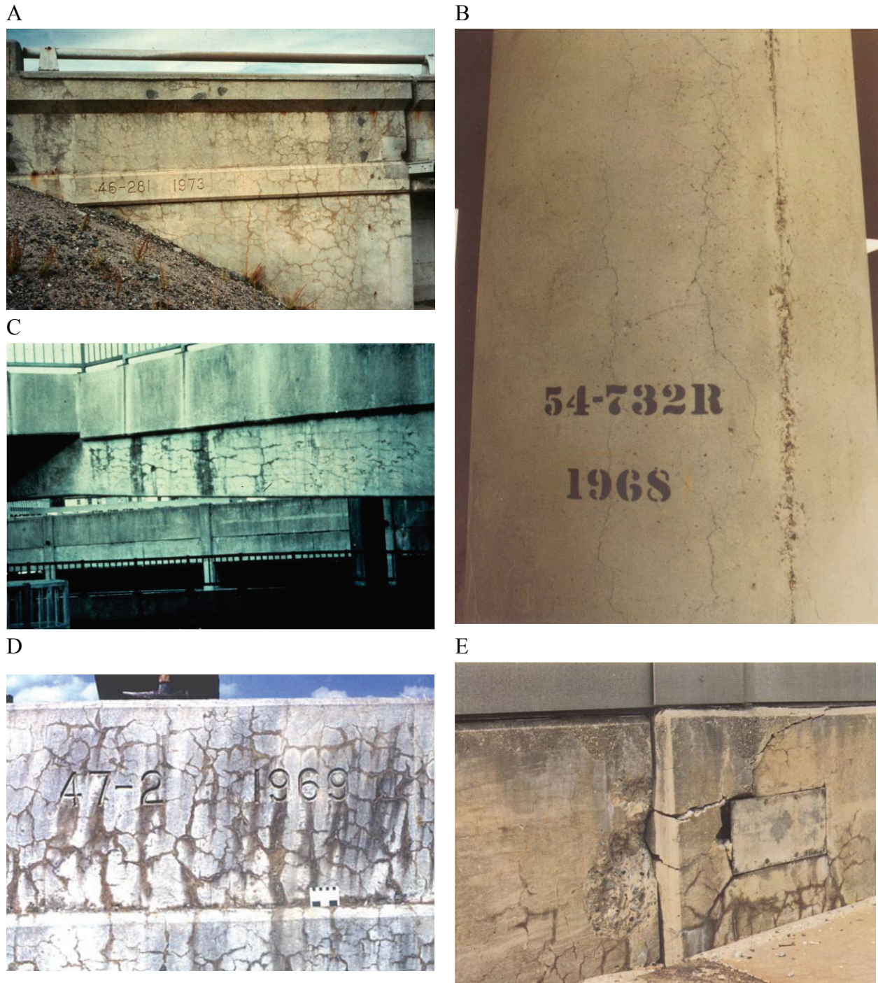
Figure 7.2. ASR-related defects in bridge elements and severity assessment. A. Map cracking on bridge abutment (condition state 3). B. Aligned cracking on column (condition state 2). C. Aligned cracking in beam (condition state 3). D. Gel exudation (condition state 3). E. Relative dislocation/misalignment, leading to loss of clearance and cracking (SHRP C-315 1991) (condition state 3).
