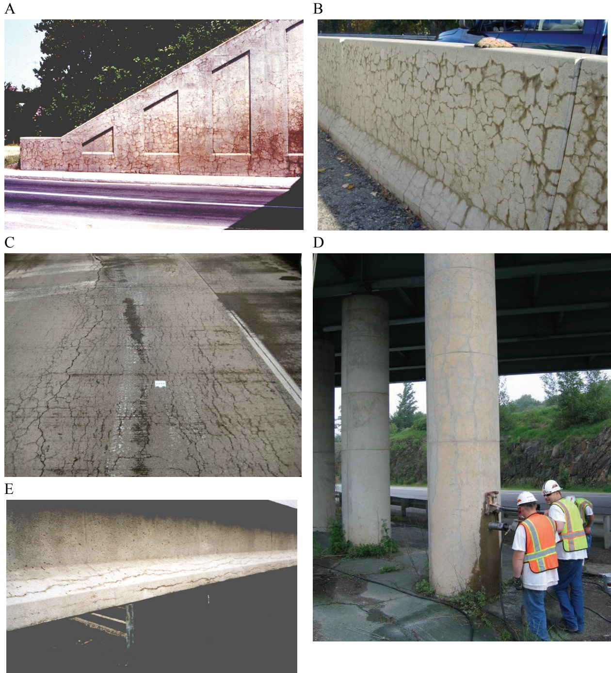
Figure 3.1. (A). Map-cracking in the wing wall of a 30-year-old bridge structure affected by ASR (CSA 2000). (B). Severe map-cracking and associated gel staining around cracks in a median highway barrier affected by ASR. (C). Well-defined crack pattern associated with the development of ASR in highway pavement; the orientation of predominant cracks is longitudinal, while map- or pattern-cracking is also identified. (D). Preferred alignment of cracks in an ASR-affected concrete column. (E). Longitudinal cracking in a precast, reinforced concrete beam affected by ASR.
