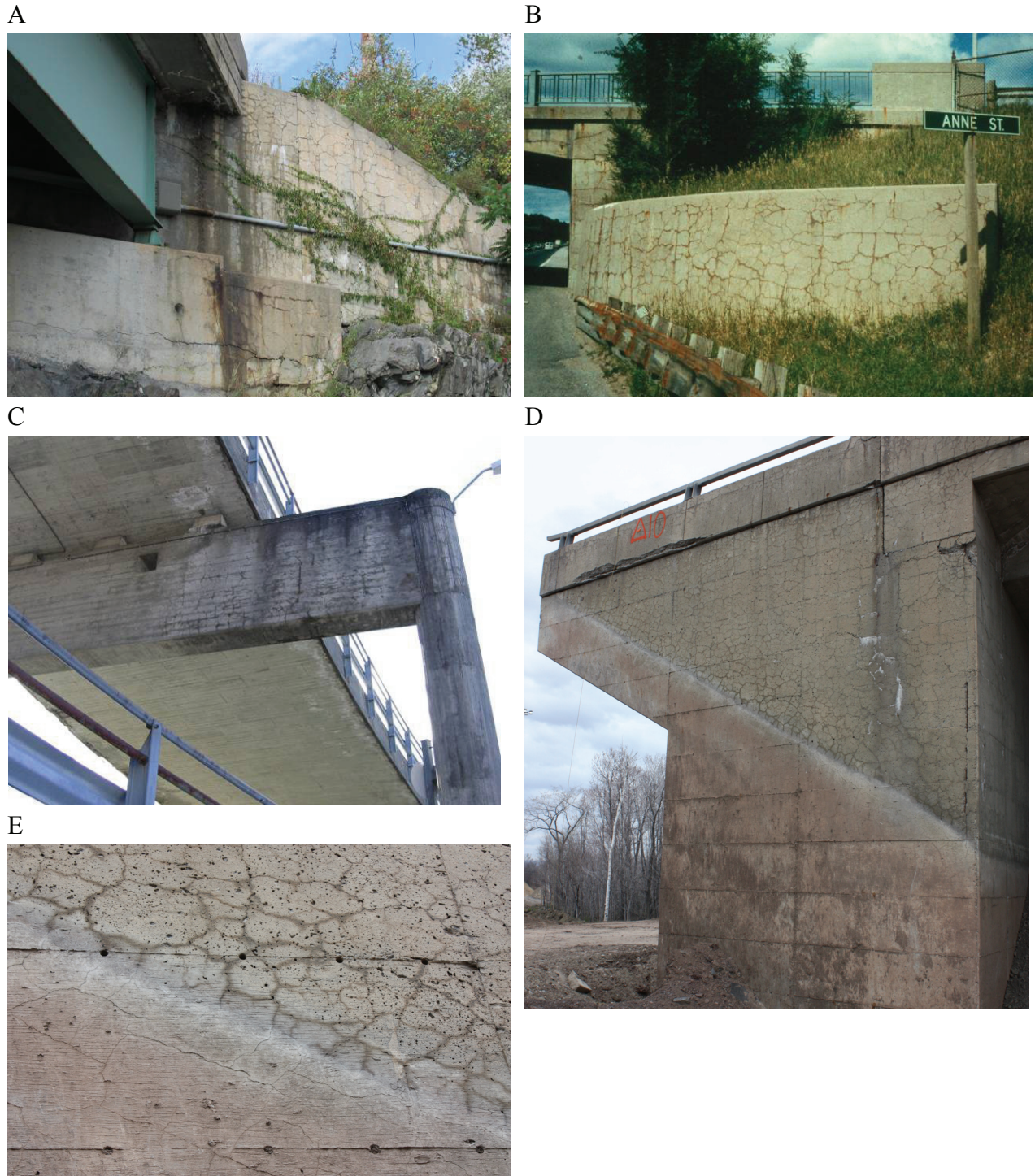
Figure 3.2. (A&B). Map-cracking in wing walls (exposed elements) of bridge structures affected by ASR. (C). Cracking in the column and the exposed portion of a beam affected by ASR. (D&E). Cracking in the exposed portion (above ground) of the wing wall of a bridge structure affected by ASR; the wing wall has been excavated before being demolished. The lower ground portion shows limited cracking; discoloration occurs around the cracks above ground (E).
