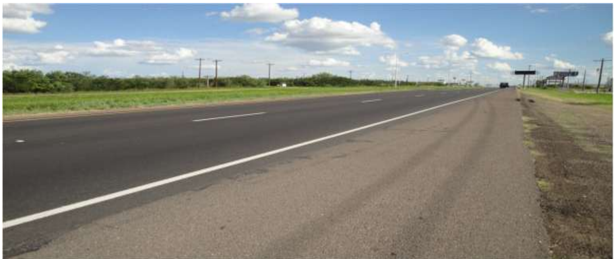
Figure III-5. Example Completed 2" Thick HMA Mat on US83. (4.8%PG 70-22 + Crushed Gravel + 20% RAP + 1% Lime)
