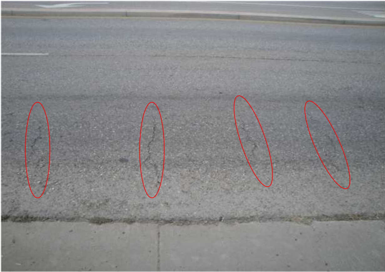
Figure II-2. Example of Cracking on US 59 Prior to 2" HMA Overlay.
