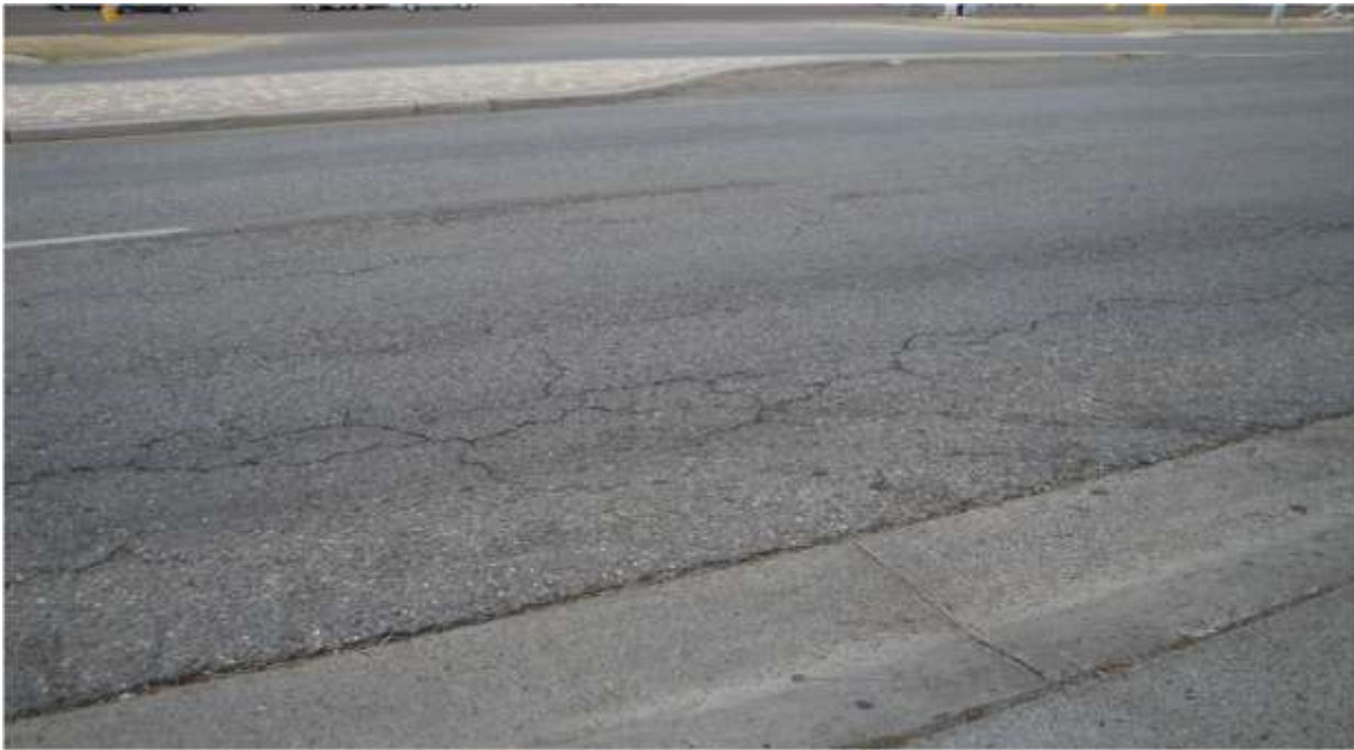
Figure II-3. Example of Cracking on US 59 Prior to 2" HMA Overlay.
