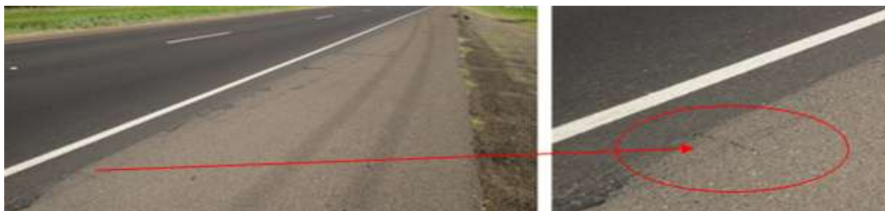
Figure II-1. Example of Cracking on US 83.
