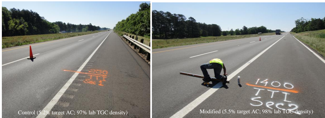
Figure II-3. View of the Test Sections – No Visible Surface Rutting (After 1 Year; May 2011).
