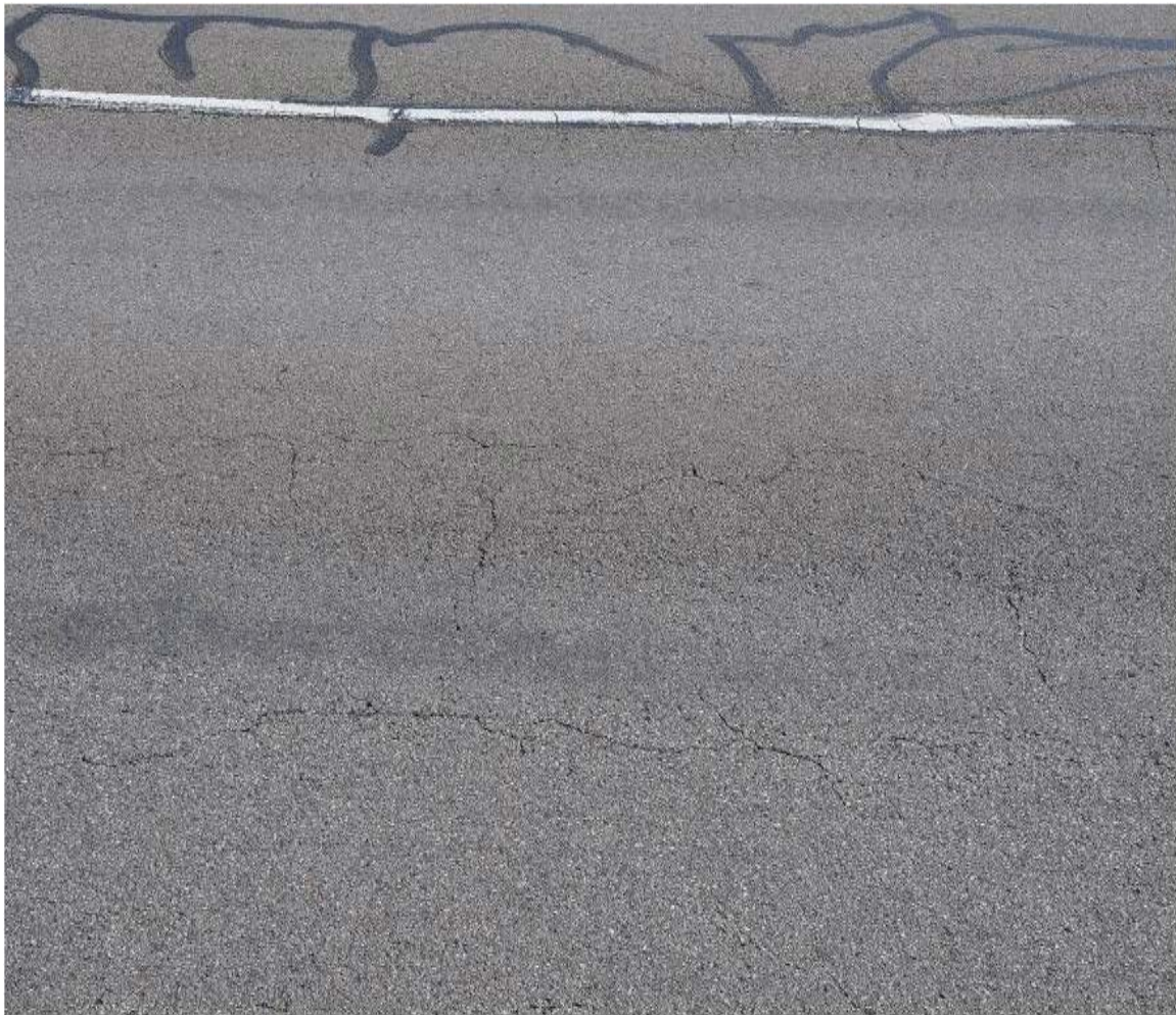
Figure 4. Example of Cracks on Control Section 01.
