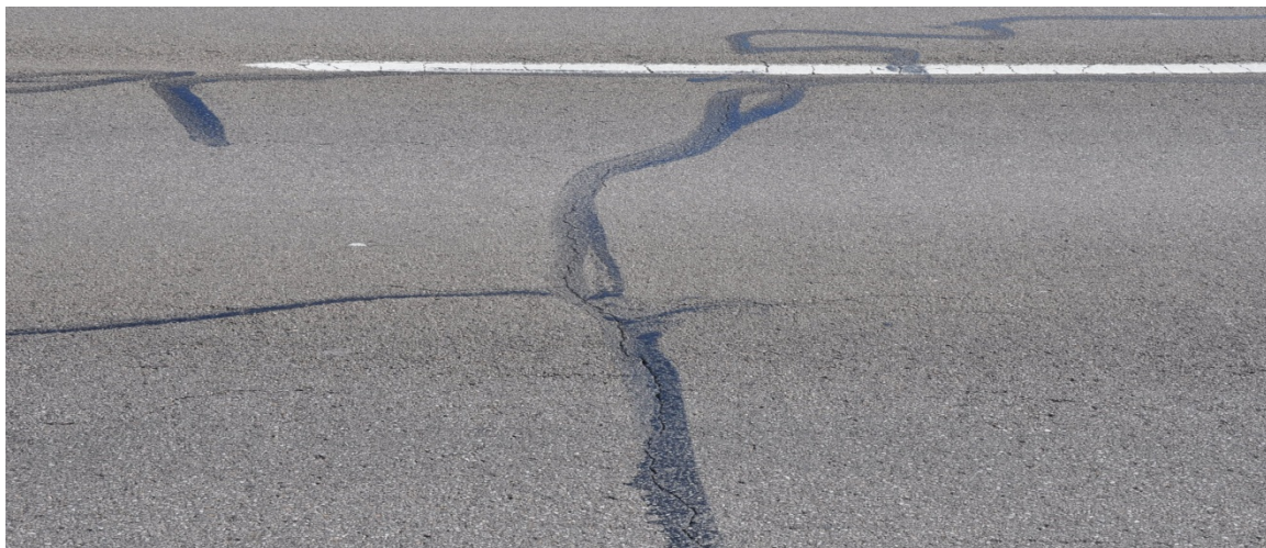
Figure 7. Example of Severe Cracks on Modified Section.
