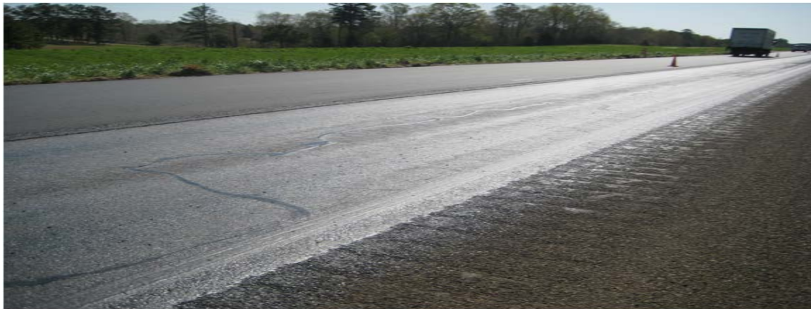
Figure 9. Example of Transverse cracks in Section 02.
