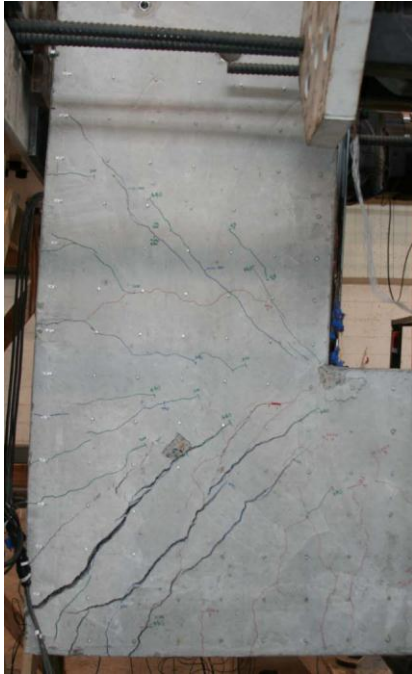
(a) Photograph of crack pattern at incipient failure near end of experiment.
