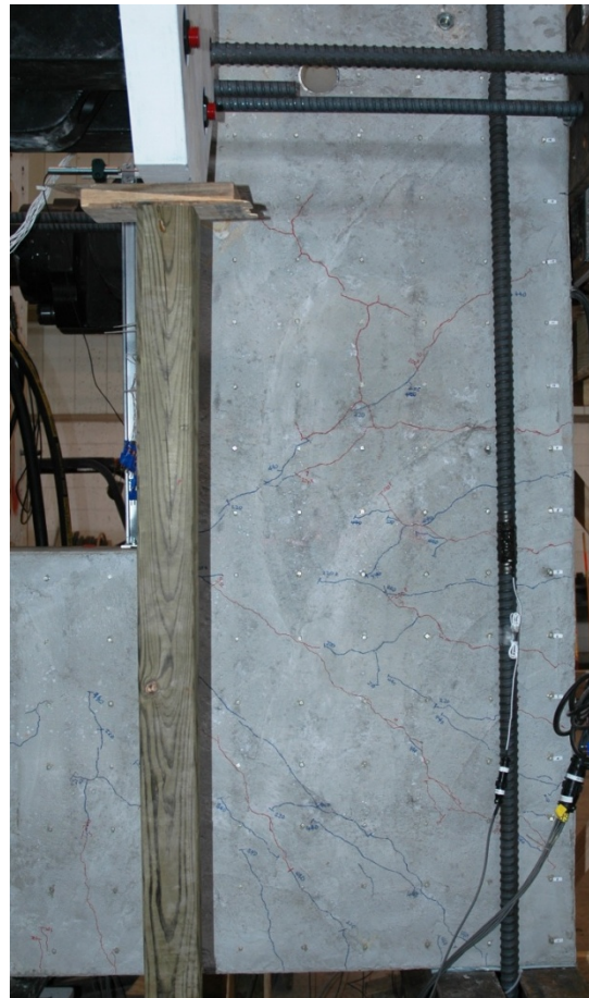
(b) Singly reinforced beam
