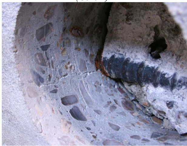
(c) Crack from the surface to reinforcing steel (Core 2)
