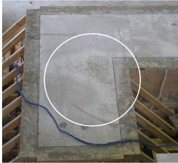
(a) Map-cracking due to thermal effect
