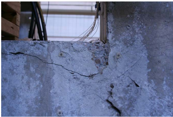
(c) Crush cover at the interior corner of the joint
