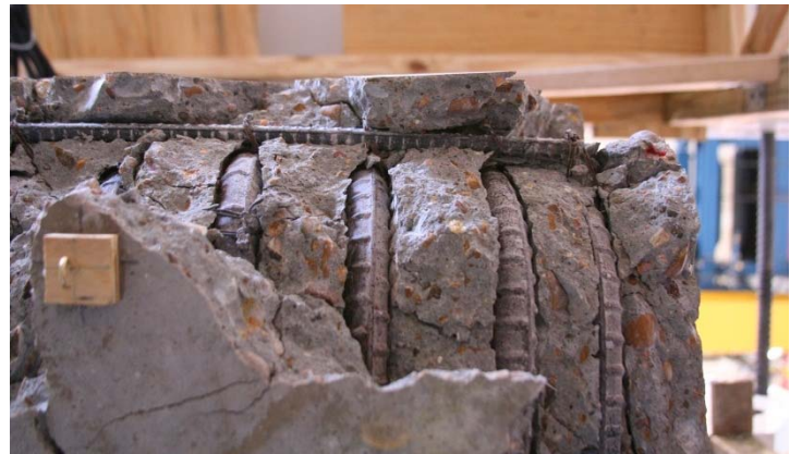
(f) Exterior face of the beam-column joint showing bulging of the U-bars and laterally displaced longitudinal steel
