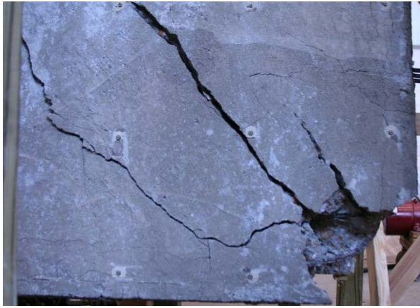
(a) Failure at the exterior corner
