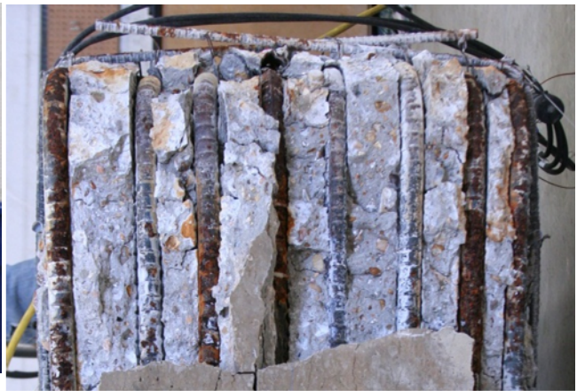
(f) Exterior face of the beam-column joint showing bulging of the U-bars, laterally displaced longitudinal steel, and reinforcing steel corrosion
