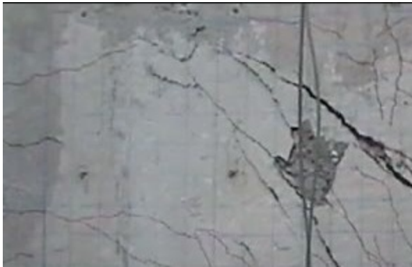
(c) Crush cover at the interior corner of the joint
