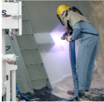
A TEERM team member applies a thermal spray coating on a Launch Structure at KSC, to test the effectiveness of coatings low in volatile organic compounds.
