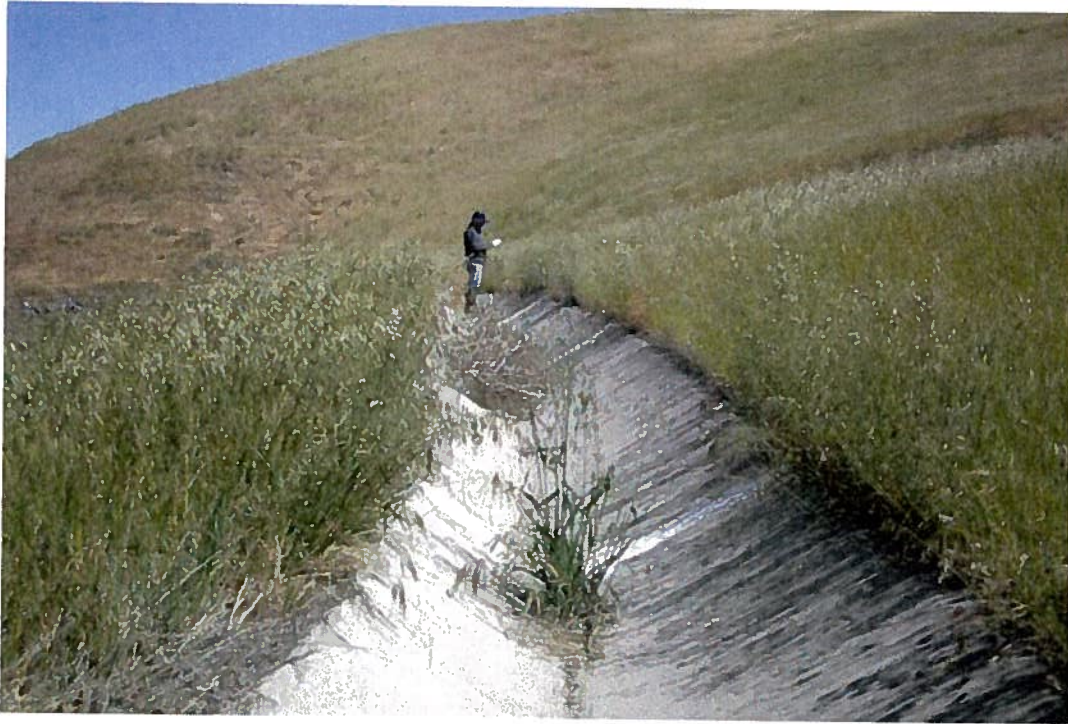
Figure 5 Building 829 Landfill Vegetative Debris Accumulation and Growth in Concrete Drainage Ditch
