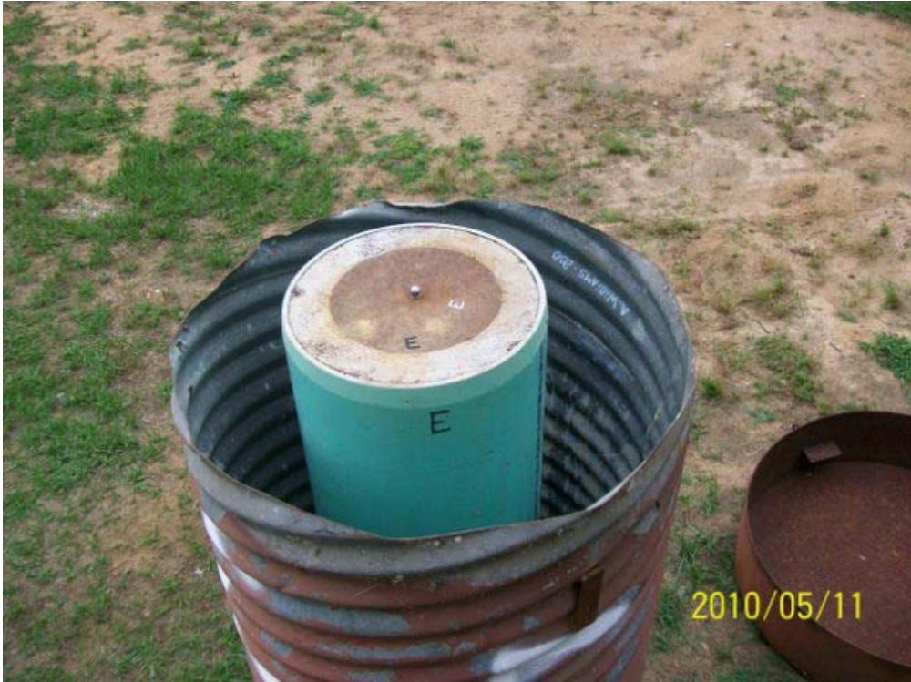
Figure 4-1c. Monument pedestal in soil (Savannah Bluff Lock and Dam – photo by Joyner Keeny, PLLC)
