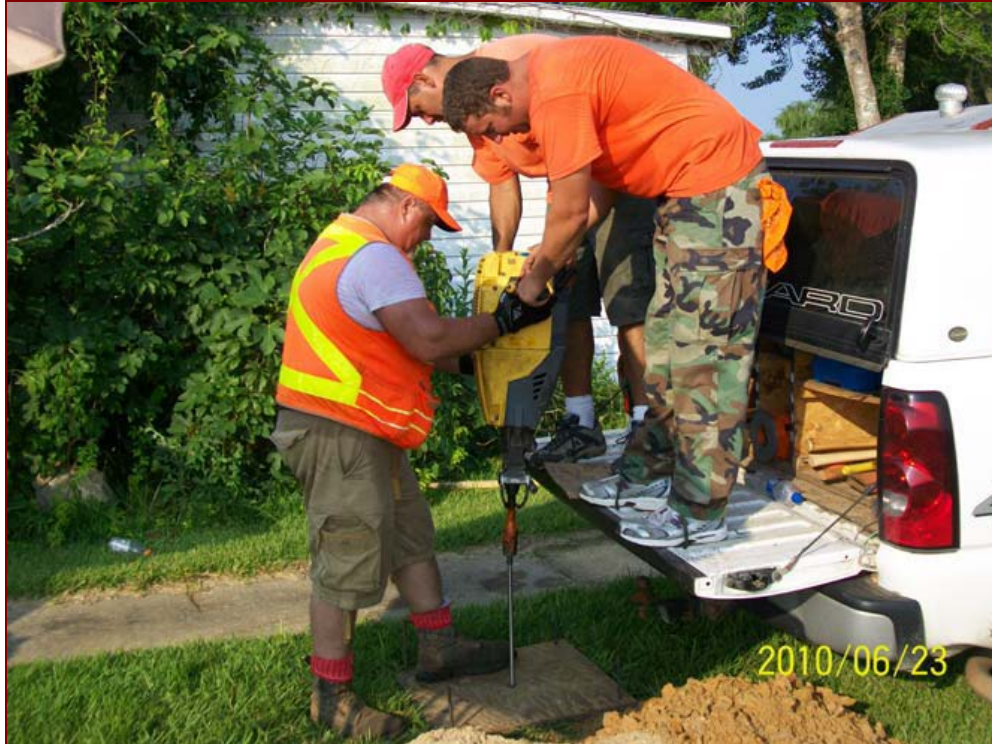
Figure 3-3. Driving a stainless steel rod with the Cobra Combi driving jackhammer Wilmington District (2010)
