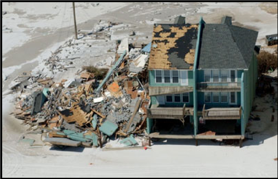
Navarre Townhouse after Hurricane Ivan, September 2004 (courtesy of PensacolaNews.com 2004)
