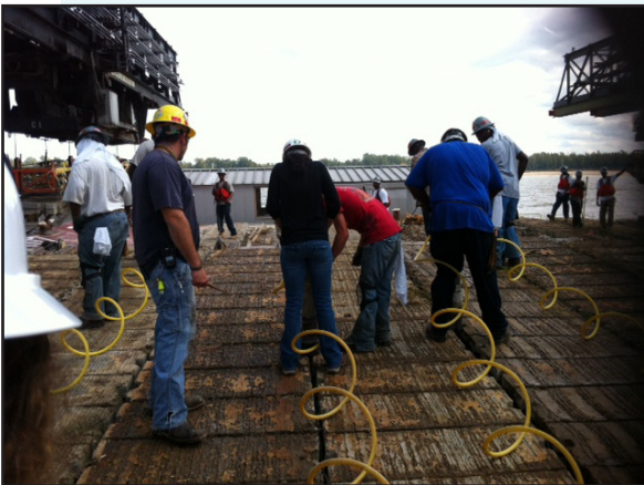
VLDP members get close up view of the MSU crew at work.
