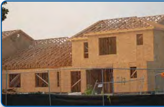
A junior-enlisted multiplex under construction at Dover Air Force Base. At project completion in 2009, the 212 homes constructed in 2004 - 2005 will be joined by 768 new homes.
