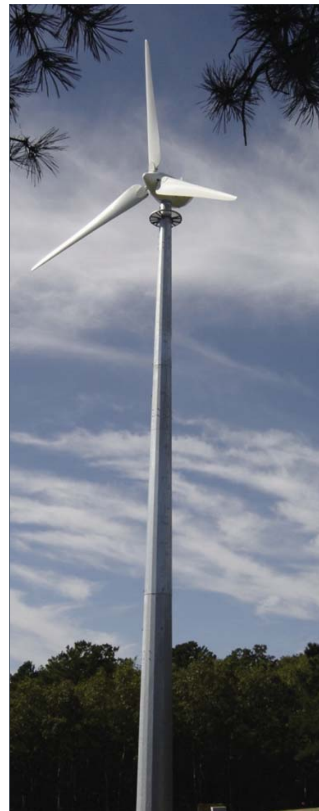
50 kW wind turbine at Bourne National Cemetery will supply virtually all of the cemetery's annual electricity.
