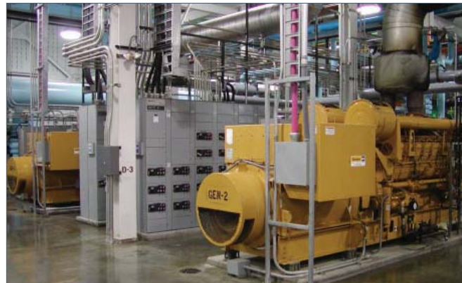
New cogeneration systems will produce similar benefits to the existing plant at the Mt. Home VA Medical Center.
