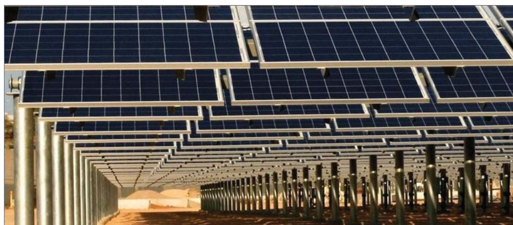
Crystalline silicon photovoltaic modules recently installed at the Southern Arizona VA Medical Center.
