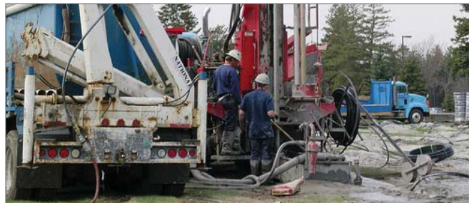
Nearly all the bore holes are complete for the ground source heat pump system at St. Cloud VA Medical Center.
