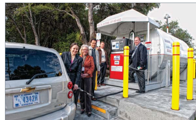
The Martinez campus uses E-85 fuel from this station in its 103 flexible fuel vehicles.
