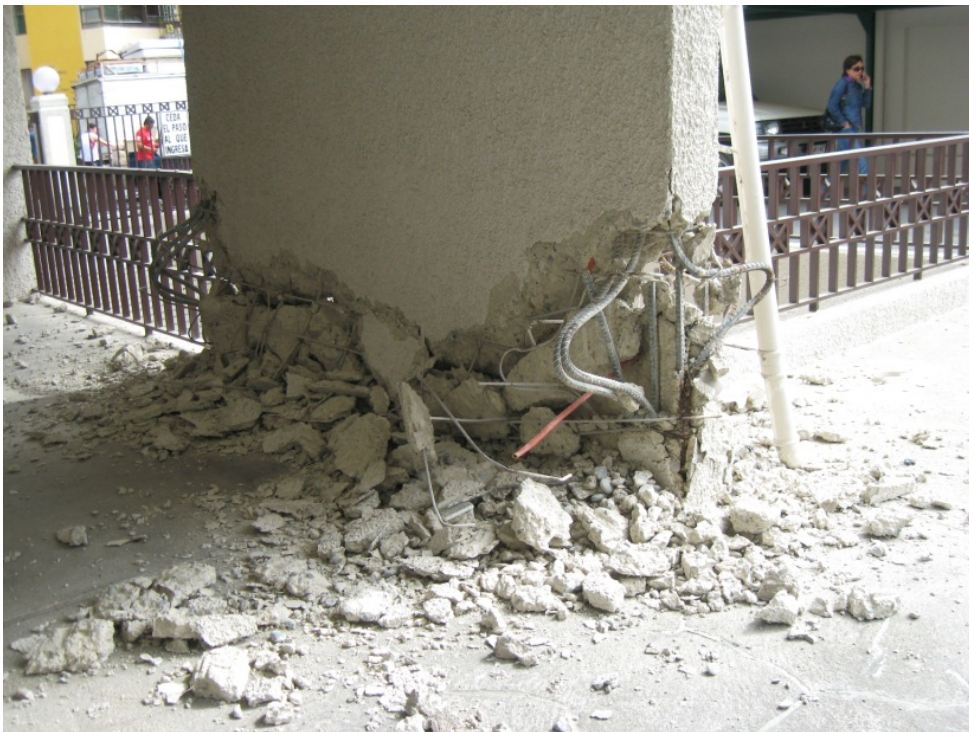
Figure 5-7 Crushing and bar buckling in the transverse shear wall on Line 1 resulting in significant differential vertical displacement (photo courtesy of Patricio Bonelli).
