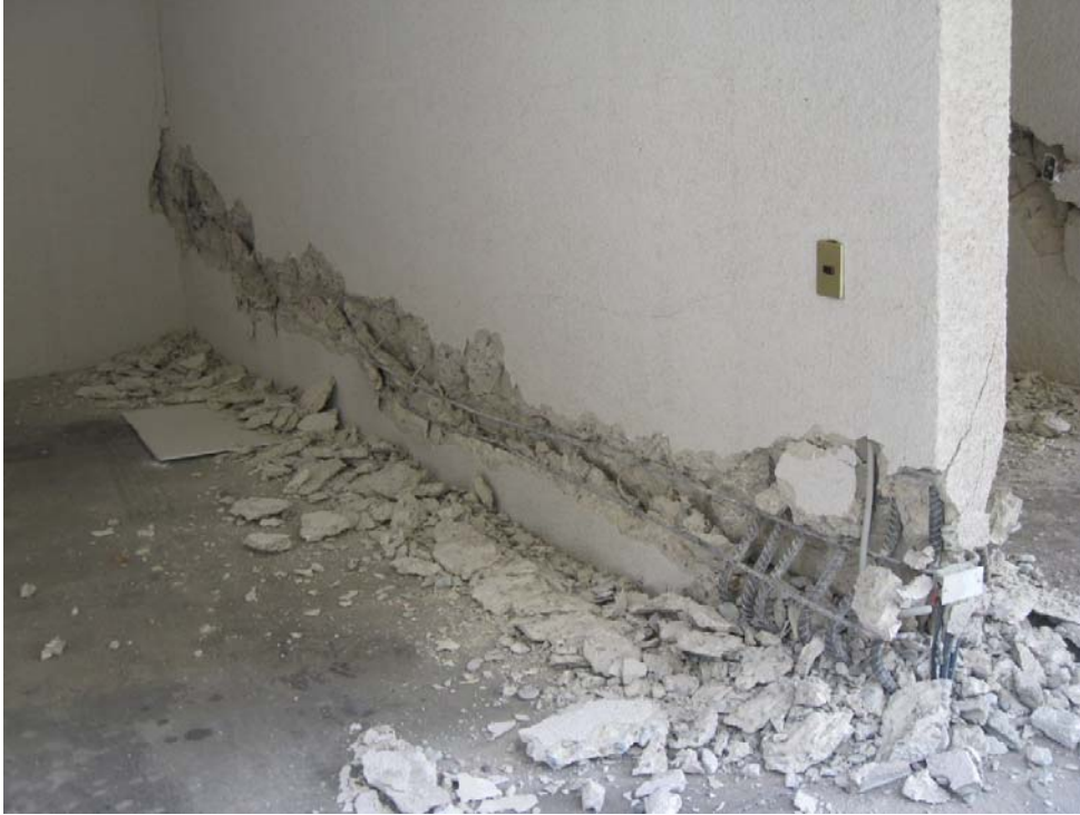
Figure 5-6 Cracking, spalling, crushing, and bar buckling in the transverse shear wall on Line 5 (photo courtesy of Patricio Bonelli).
