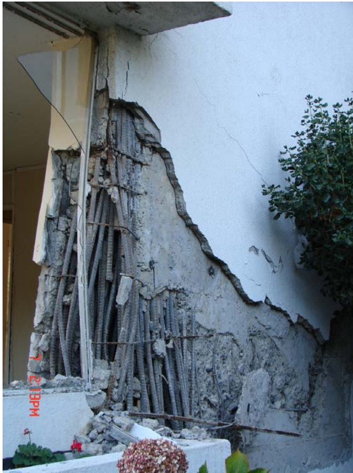
Figure 2-7 Damage to typical unconfined shear wall boundary zone observed in the 2010 Maule earthquake (photo courtesy of ASCE).
