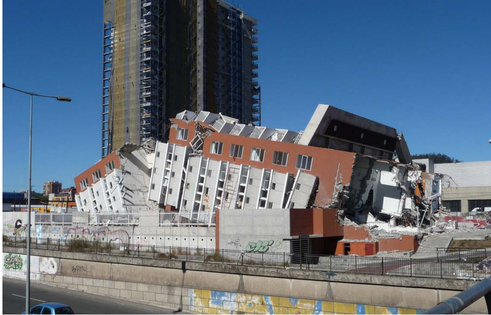
Figure 1-3 Collapse of the Alto Rio building in Concepción, Chile (photo courtesy of ATC).
