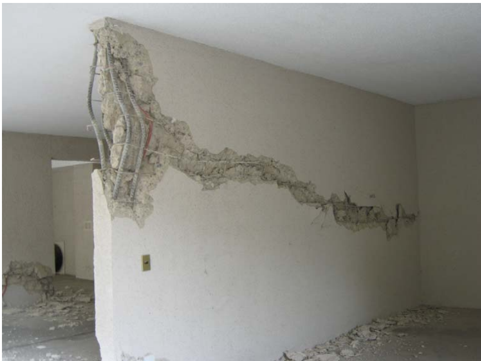
Figure 5-5 Cracking, spalling, crushing, and bar buckling in the transverse shear wall on Line 9 (photo courtesy of Patricio Bonelli).
