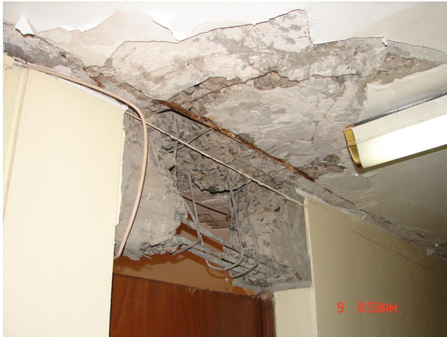
Figure 2-5 Shallow lintel showing nominal reinforcement and lack of confinement in a residential building that was damaged in the 2010 Maule earthquake (photo courtesy of ASCE).
