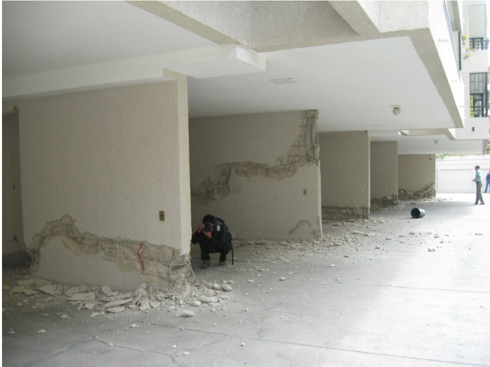
Figure 5-4 Overall damage sustained in the first-story transverse shear walls of the case study building (photo courtesy of Patricio Bonelli).
