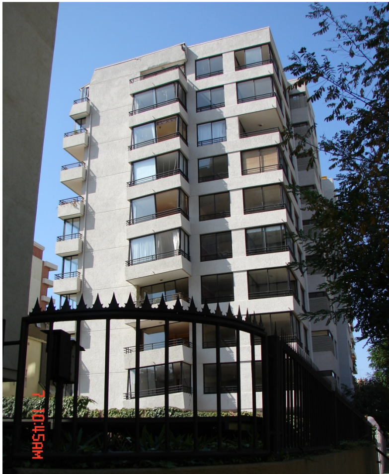
Figure 5-3 Transverse elevation of the case study building showing differential vertical displacements following the 2010 Maule earthquake (photo courtesy of Patricio Bonelli).
