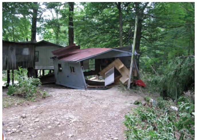
Figure 21. Views of damaged or destroyed cabins. Hydrologist pointing to high-water mark left from the June 11, 2011 flood.
