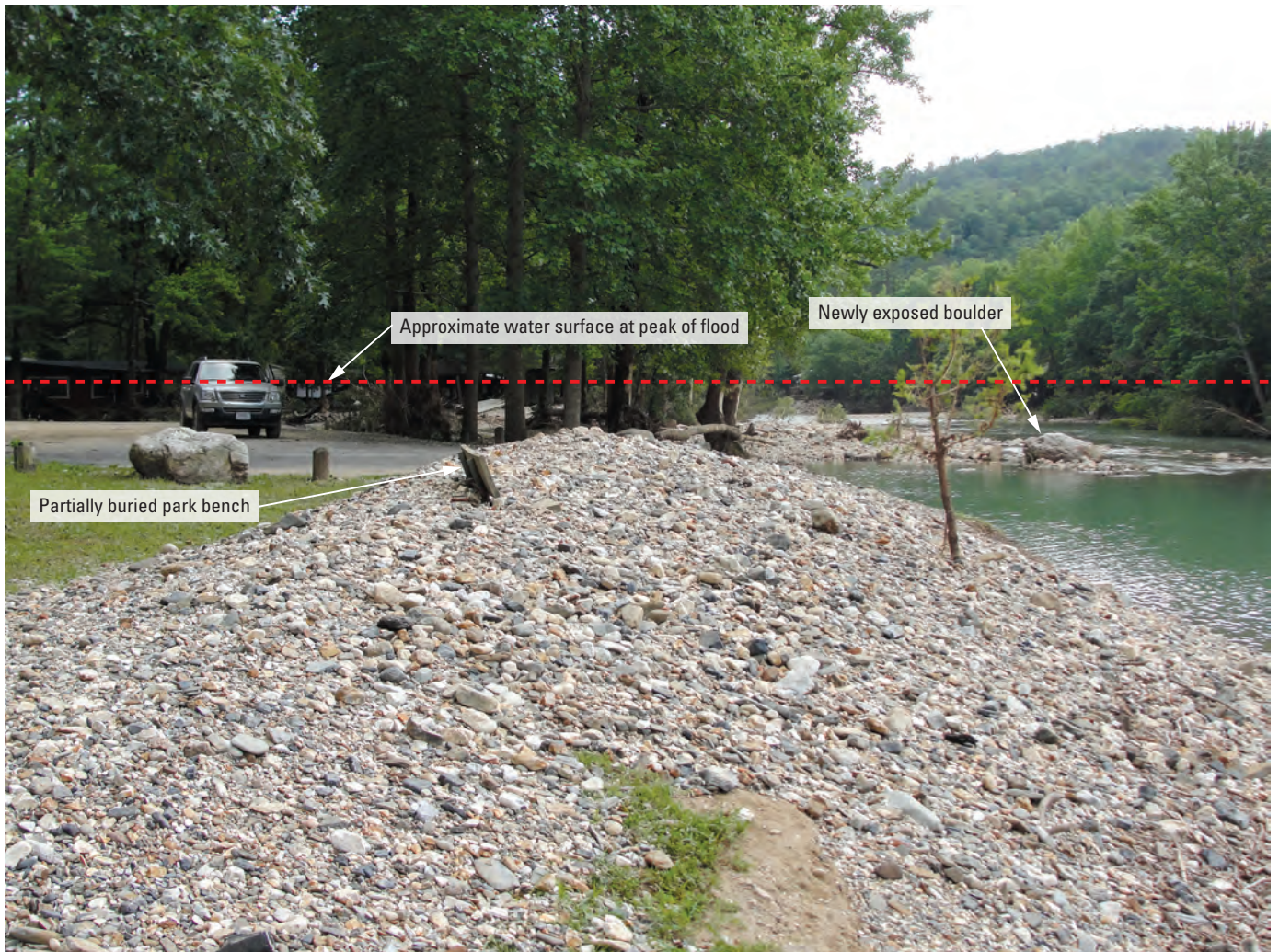
Figure 15. Downstream view of the left descending bank of the Little Missouri River along the swimming hole.
