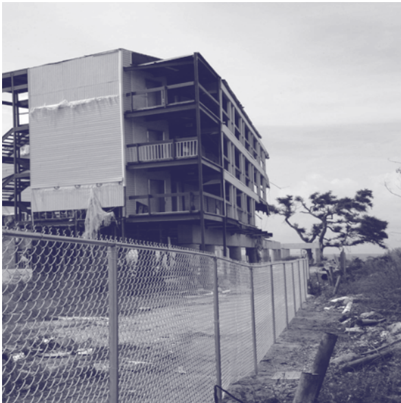
Hurricane-damaged structure along the Mississippi Gulf Coast.
