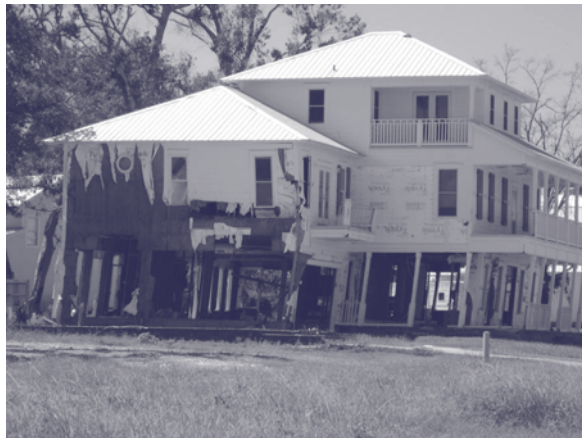
Hurricane-damaged structure along the Mississippi Gulf Coast.
