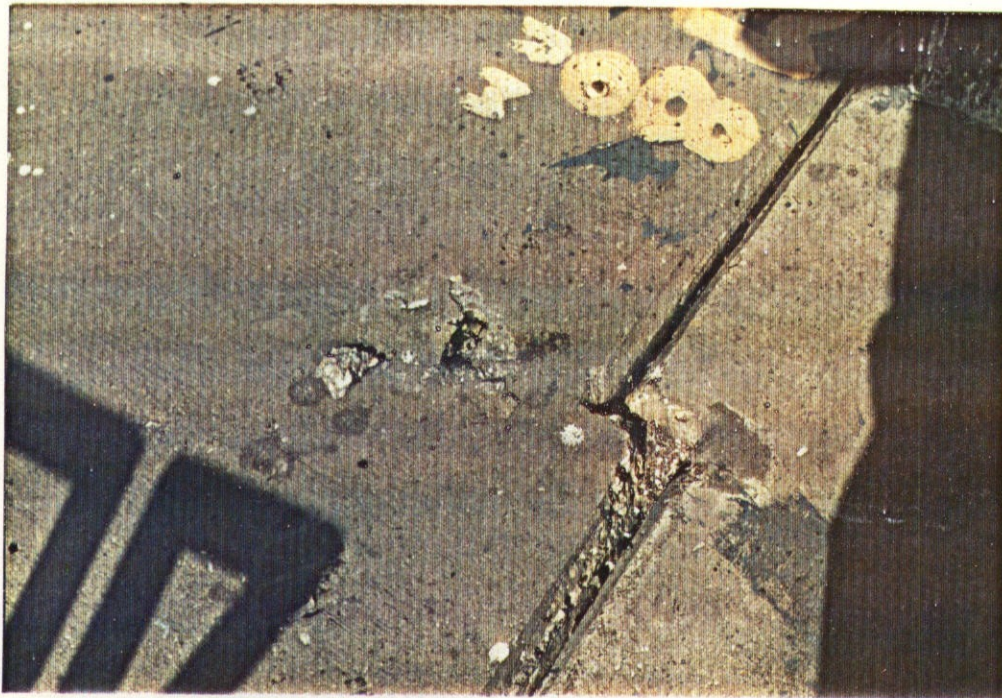
Photo 1: Concrete Popout on Top of West Side Wall
