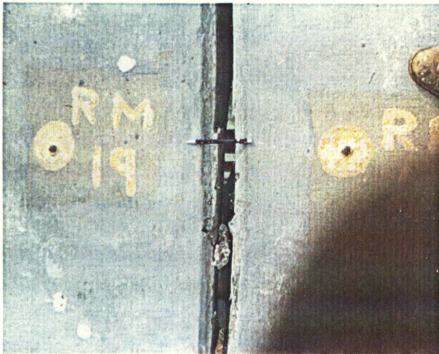
Photo 3: Excessive Gap Between RM 19 and RM 18
