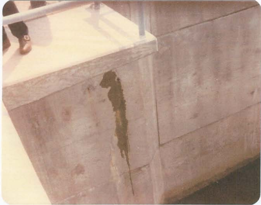
PHOTO NO. 5 - WATER LEAKING THROUGH FORM LINER BOLT HOLES
