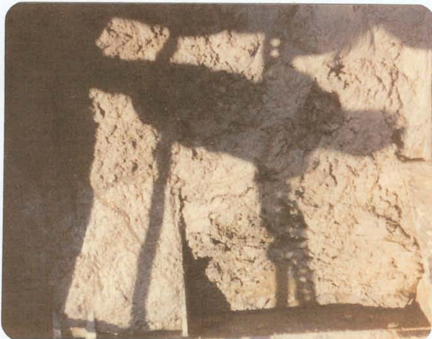
PHOTO NO. 4 - SOIL DEPOSITS IN THE GATE LIFTING RECESSES
