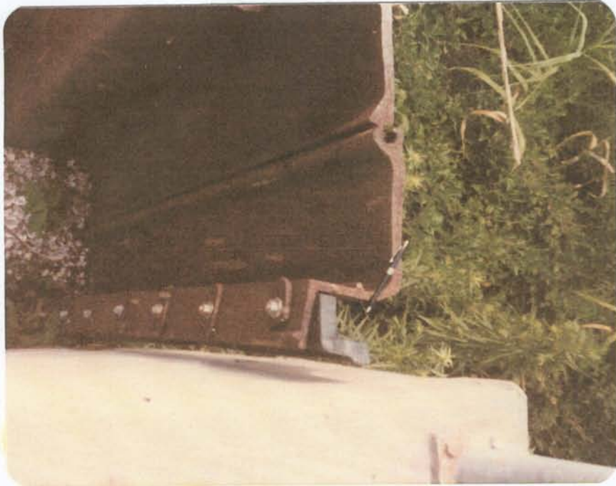
PHOTO NO. 3 - SEPARATION OF WATERSTOP BETWEEN I-WALL AND T-WALL INTERFACES
