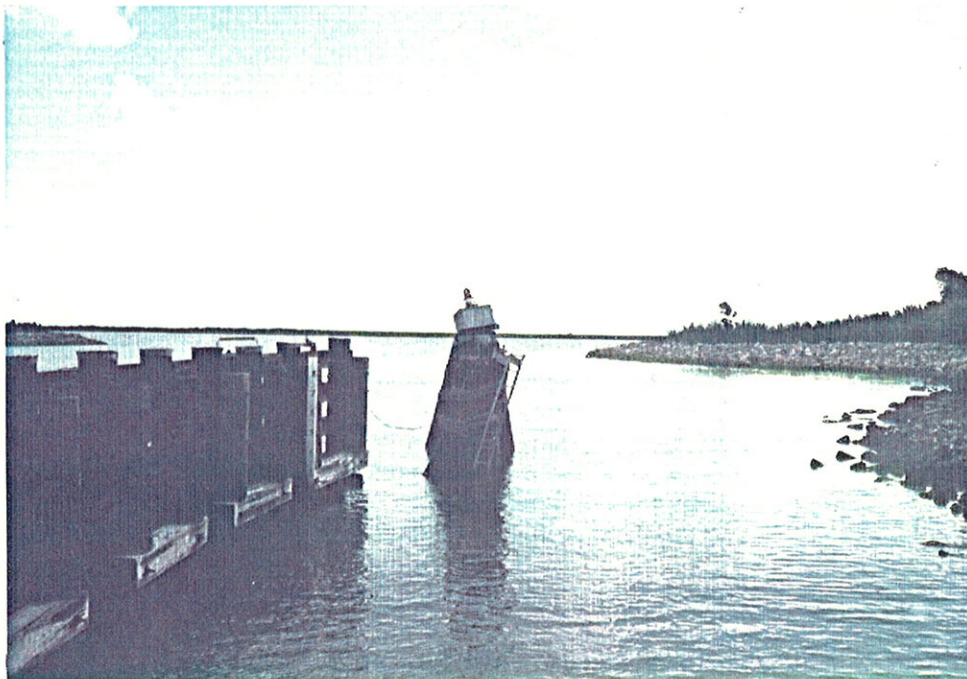
PHOTO NO. 6 - Damaged timber dolphin.
