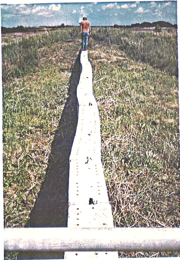
PHOTO NO. 3- Note misalignment of concrete sheetpile panels that occurred during construction.
