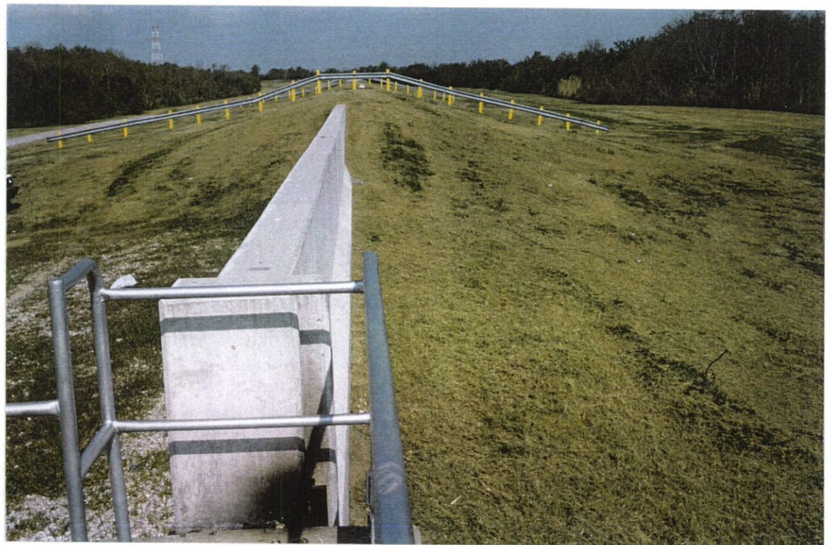
PHOTO NO. 20 – CONCRETE "I" FLOODWALL TIE IN TO LEVEE ON WEST SIDE OF STRUCTURE.
