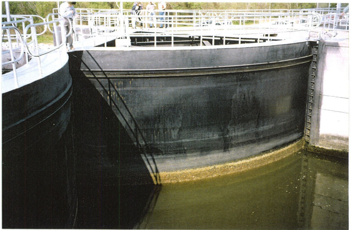
PHOTO NO. 8 – SECTOR GATE SKIN PLATE. NOTE BARNACLES AT SPLASH ZONE.
