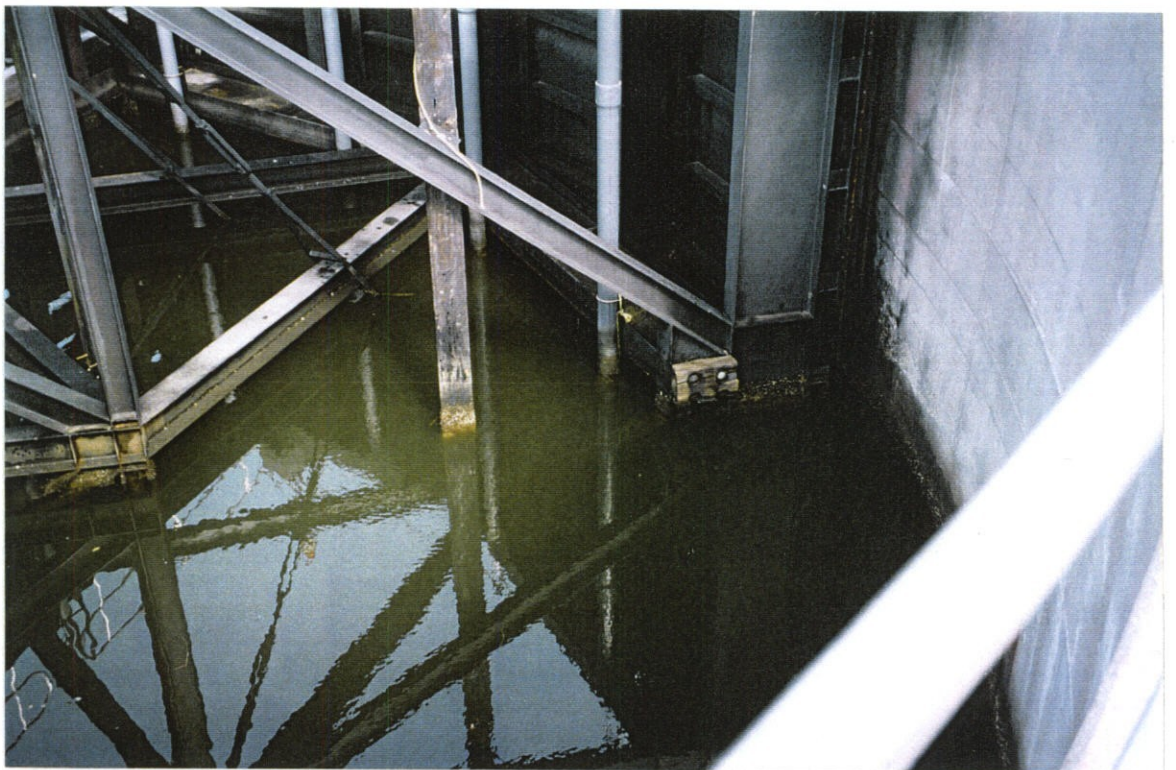
PHOTO NO. 10 – GATE SECTOR STRUCTURAL MEMBERS.
