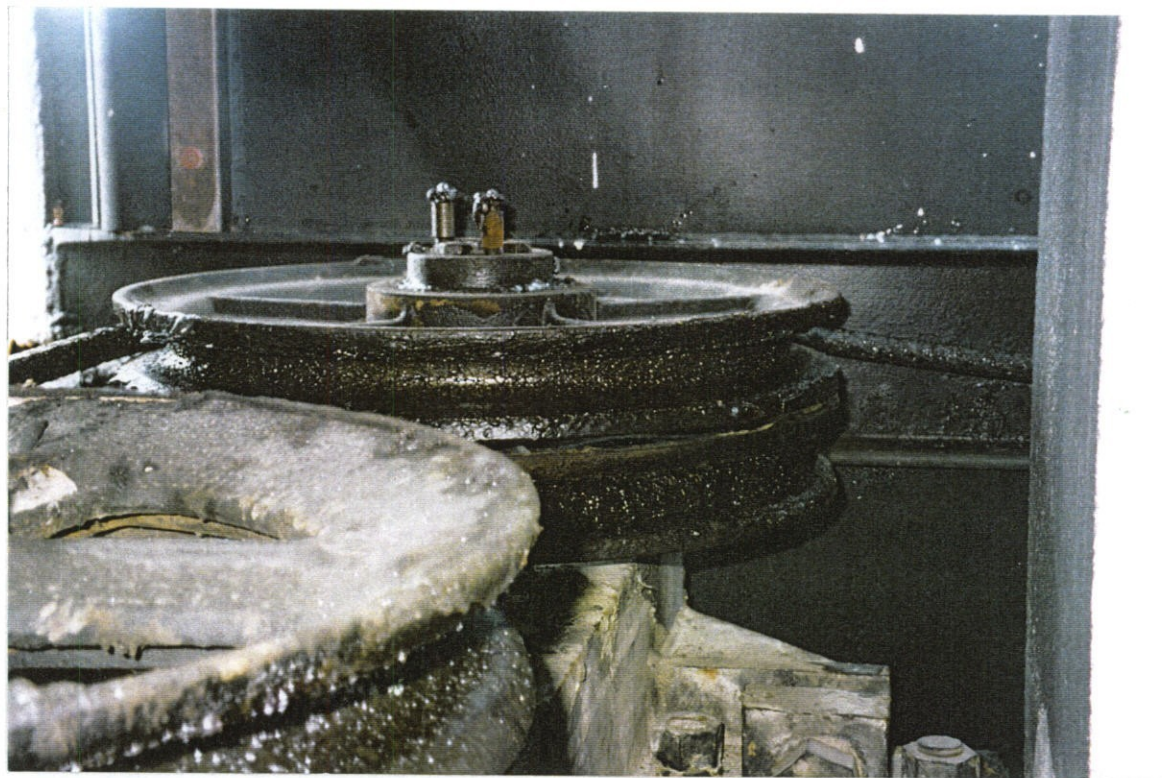
PHOTO NO. 15 – WIRE ROPE SHEAVES. NOTE SLACK CABLE.
