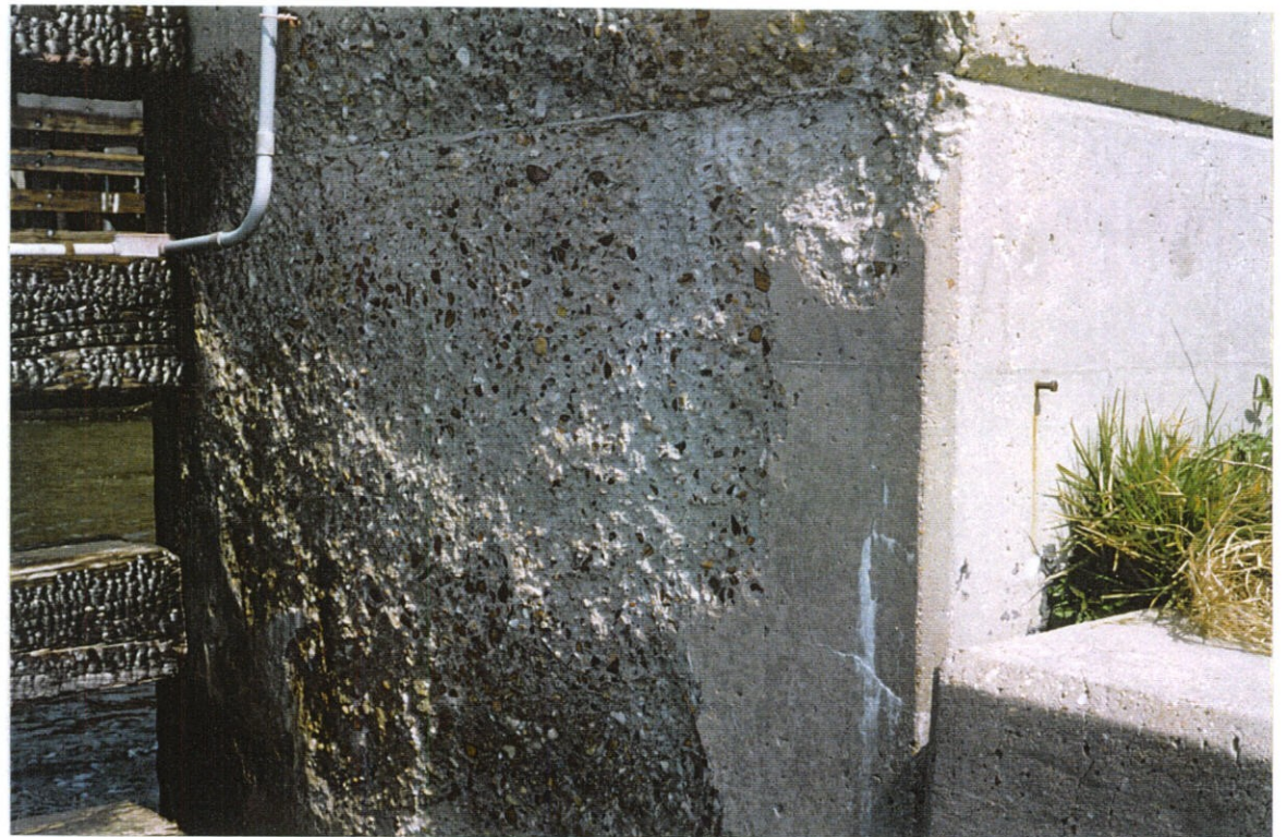
PHOTO NO. 6 – CLOSEUP OF SPALL SHOWN IN PHOTO NO. 5.
