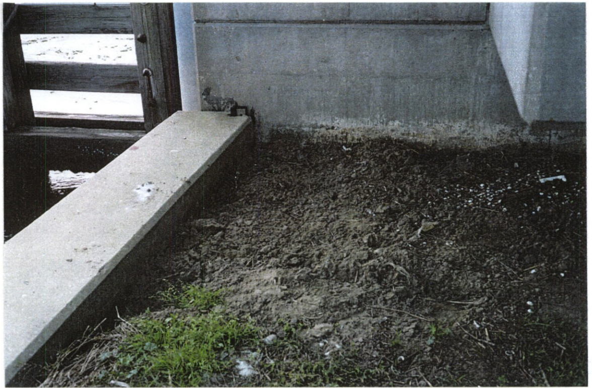
PHOTO NO. 21 – FRESH FILL BEHIND NORTHWEST WINGWALL AT ITS JUNCTURE WITH THE GATE BAY MONOLITH.
