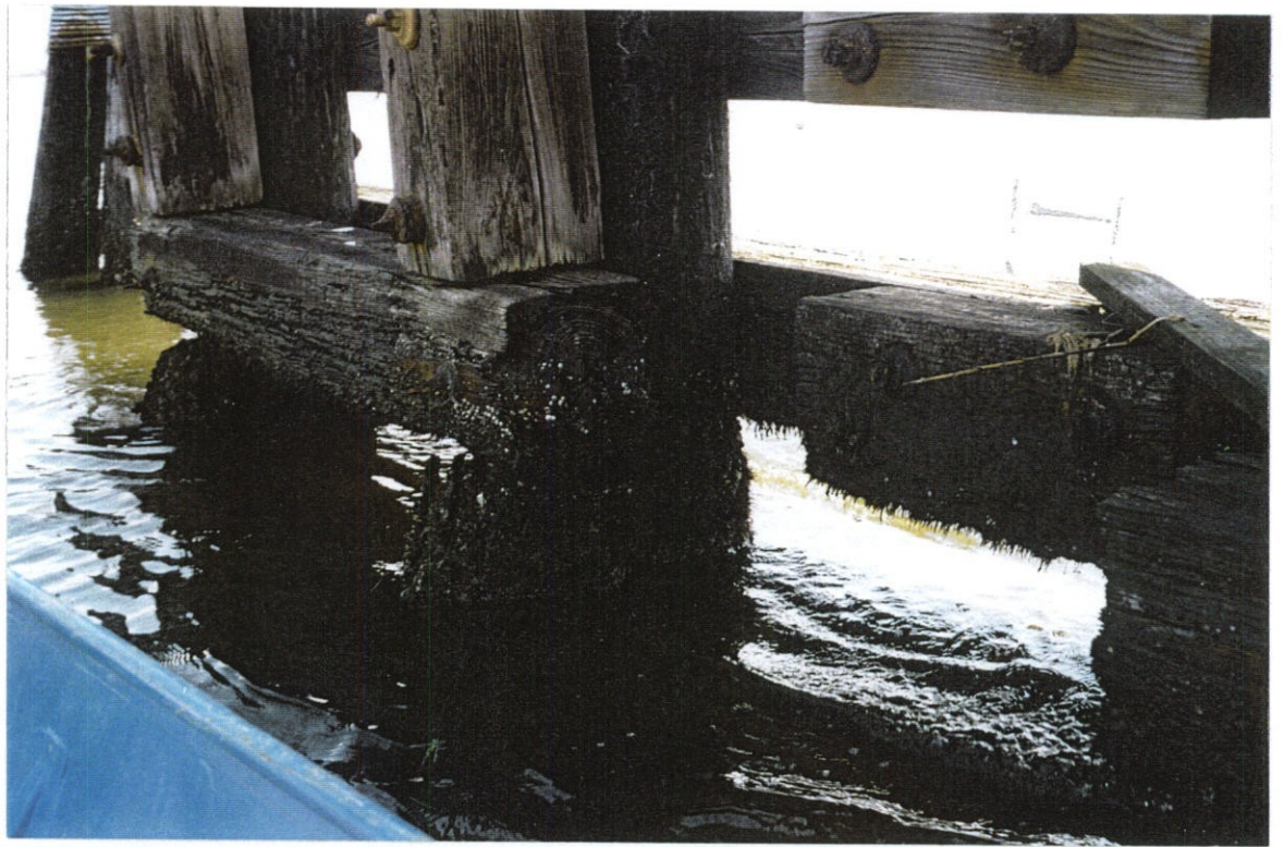
PHOTO NO. 23 – DETERIORATED HORIZONTAL GIRTS AND TOPS OF BATTERED PILES ON TIMBER GUIDEWALLS.
