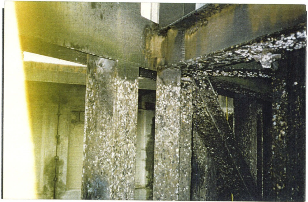
Photo 5. Marine growth on wide flange members of gate below waterline.
