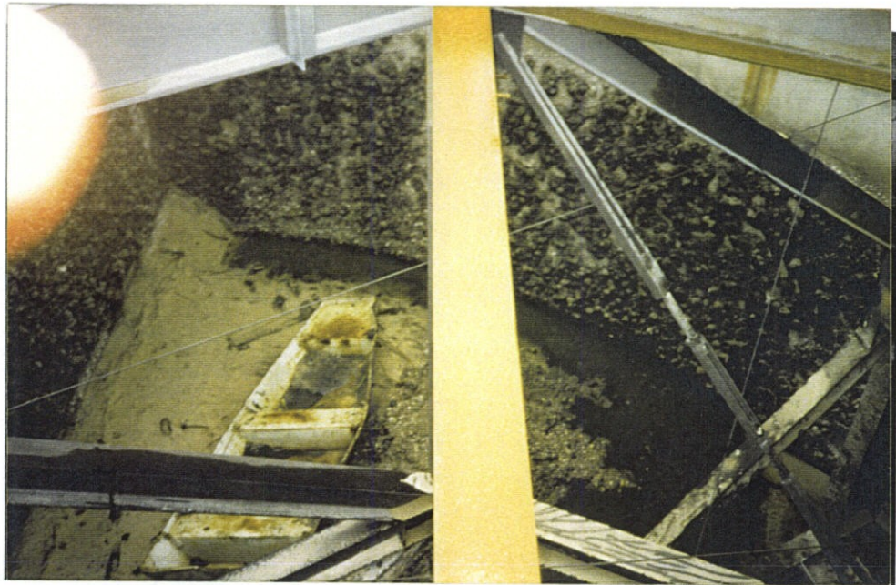
Photo 8. Gate recess area (Typical). Note silt build up against the back wall and marine growth on concrete wall.
