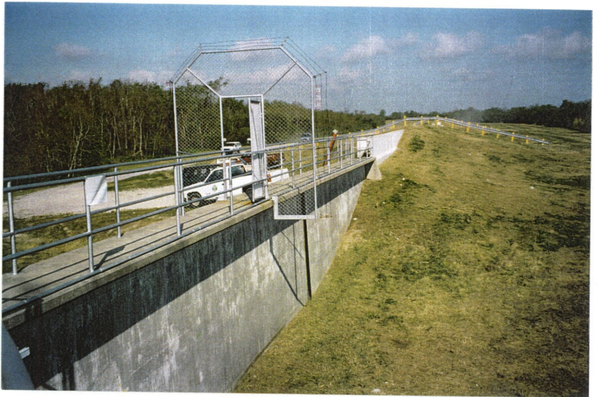
PHOTO NO. 13 – WEST "T" WALLS AND CONCRETE FLOODWALLS WITH SECURITY ACCESS GATE.
