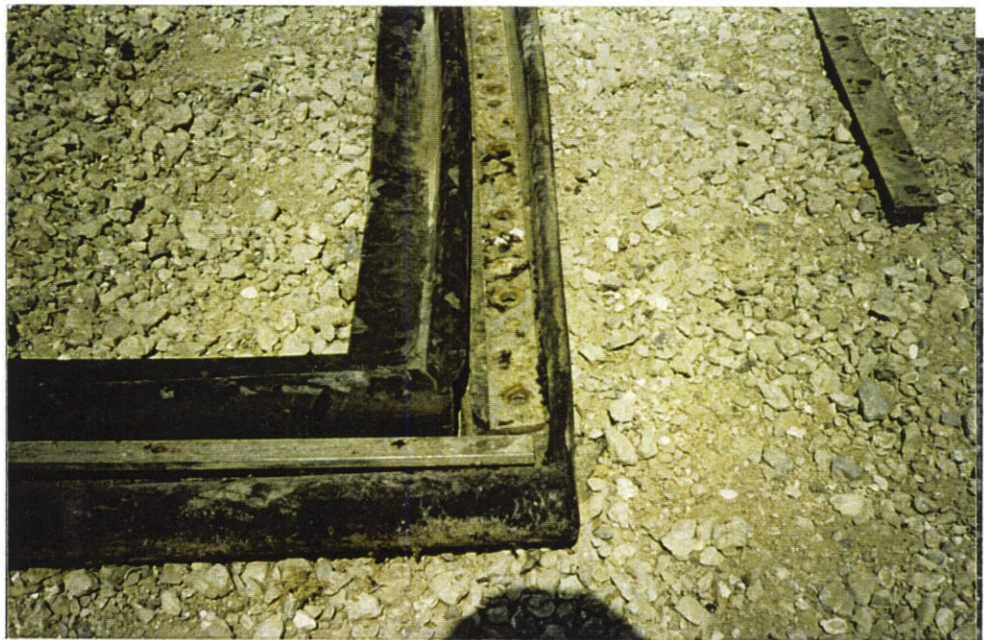
Photo 4. Sector Gate old rubber seal.
