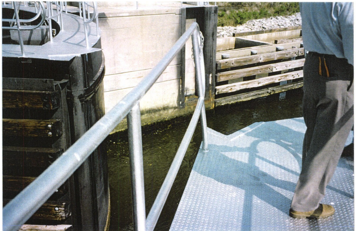
PHOTO NO. 12 – SLIGHTLY BENT HANDRAIL POST ON MITER END OF EAST GATE SECTOR.
