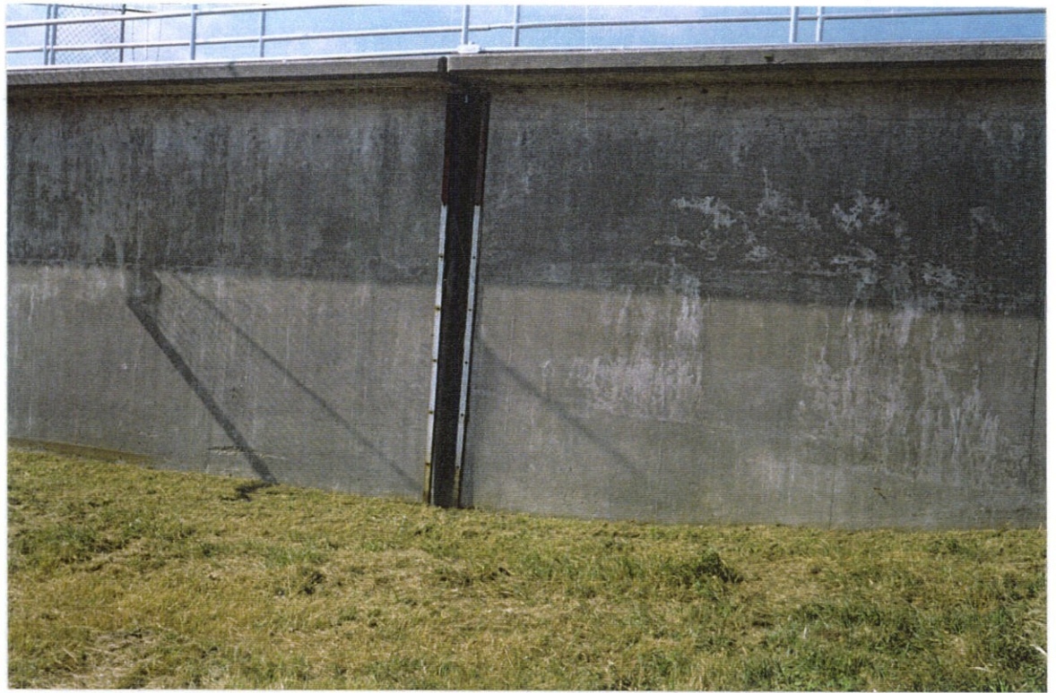
PHOTO NO. 3 - NEOPRENE SHEET OVER FLOODSIDE OF JOINT BETWEEN WEST "T" WALL MONOLITHS.
