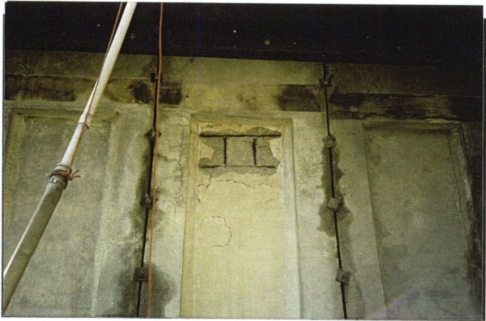
Photo 7. Spall on protected side of concrete needles with exposed reinforcing steel. Inadequate concrete cover above reinforcing steel.
