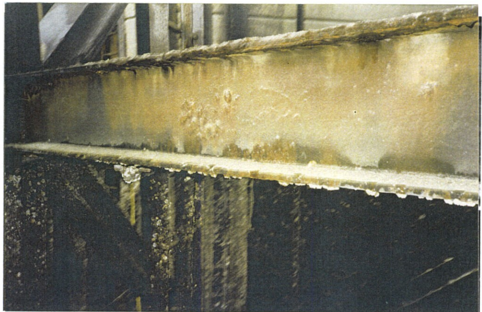
Photo 6. A wide flange member of the sector gate with corrosion.
