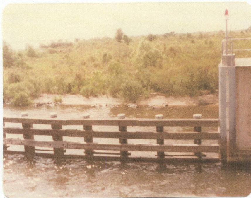
Photograph No. 8 - Missing Riprap on Bank of Approach Channel
