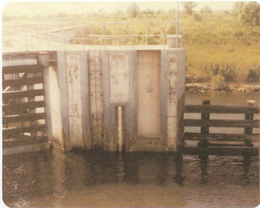
Photograph No. 5 - Rusted Structural Steel Members in Gate Bay Monolith
