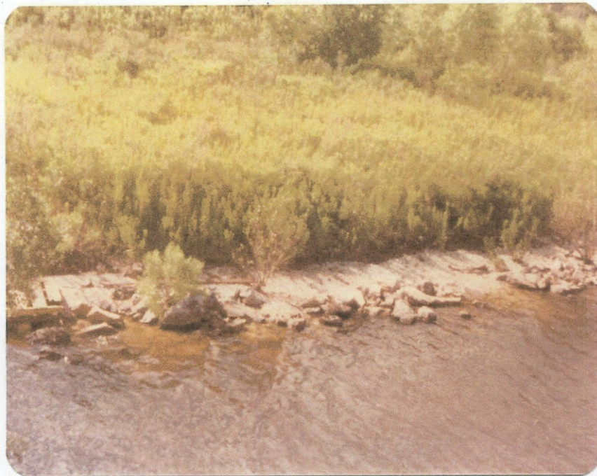
Photograph No. 7 - Missing Riprap on Bank of Approach Channel
