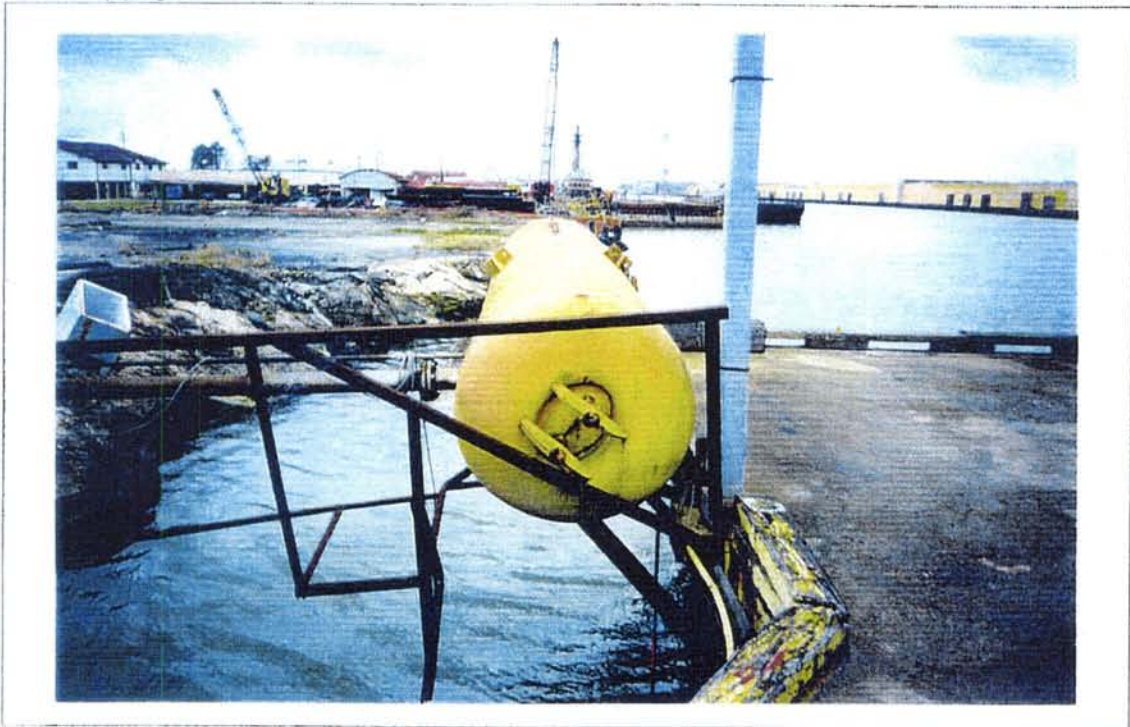
10. View to the south of the AST (Structure 41A) which was used to contain compressed air. The tank is abandoned with most of the associated piping disconnected.
