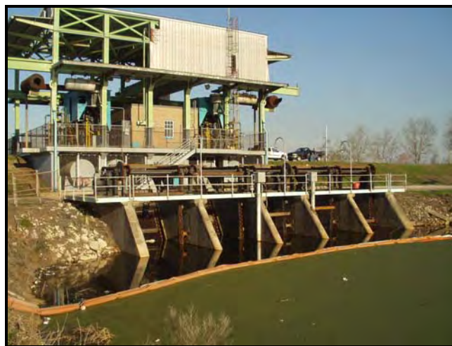
Post-Hurricane Katrina – View from the inlet canal
