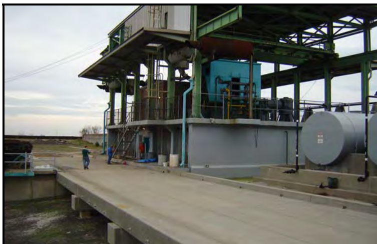
Post-Hurricane Katrina – View from the Inlet Canal
