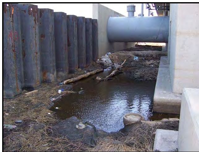
Post-Hurricane Katrina – Erosion
