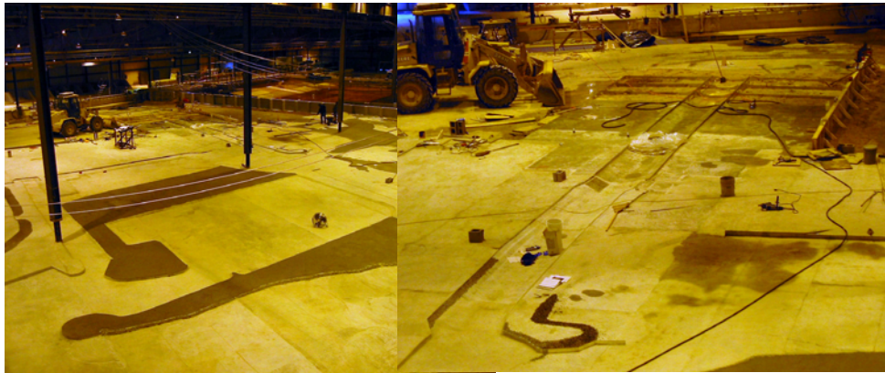
Figure V-53. Physical model during construction; left photo showing overall view, and right view looking south, down the 17th St Canal
