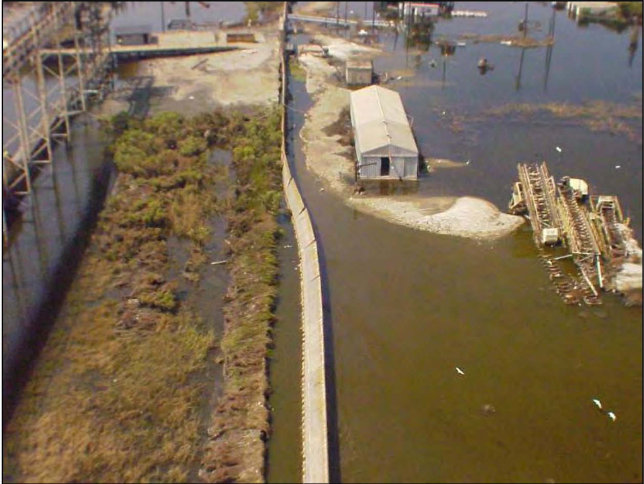
Figure 11. Katrina damaged I-wall.
