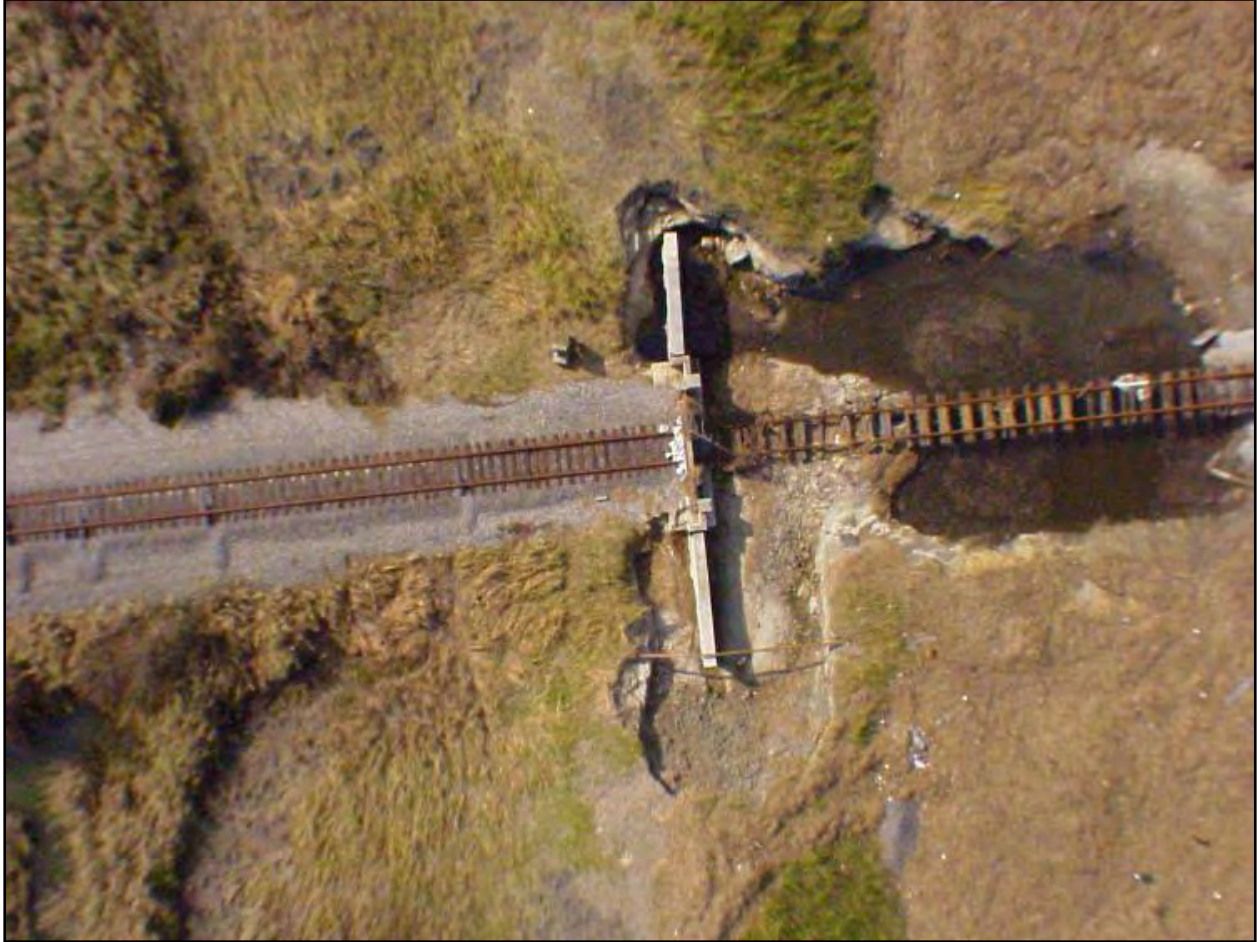
Figure 21. Katrina erosion at transition from levee to closure structure.
