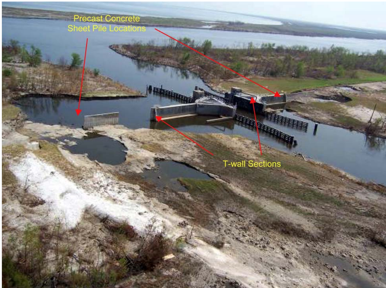
Figure STB 16. Damage at Bayou Dupre Control Structure (note breached section of precast concrete pile wall)
