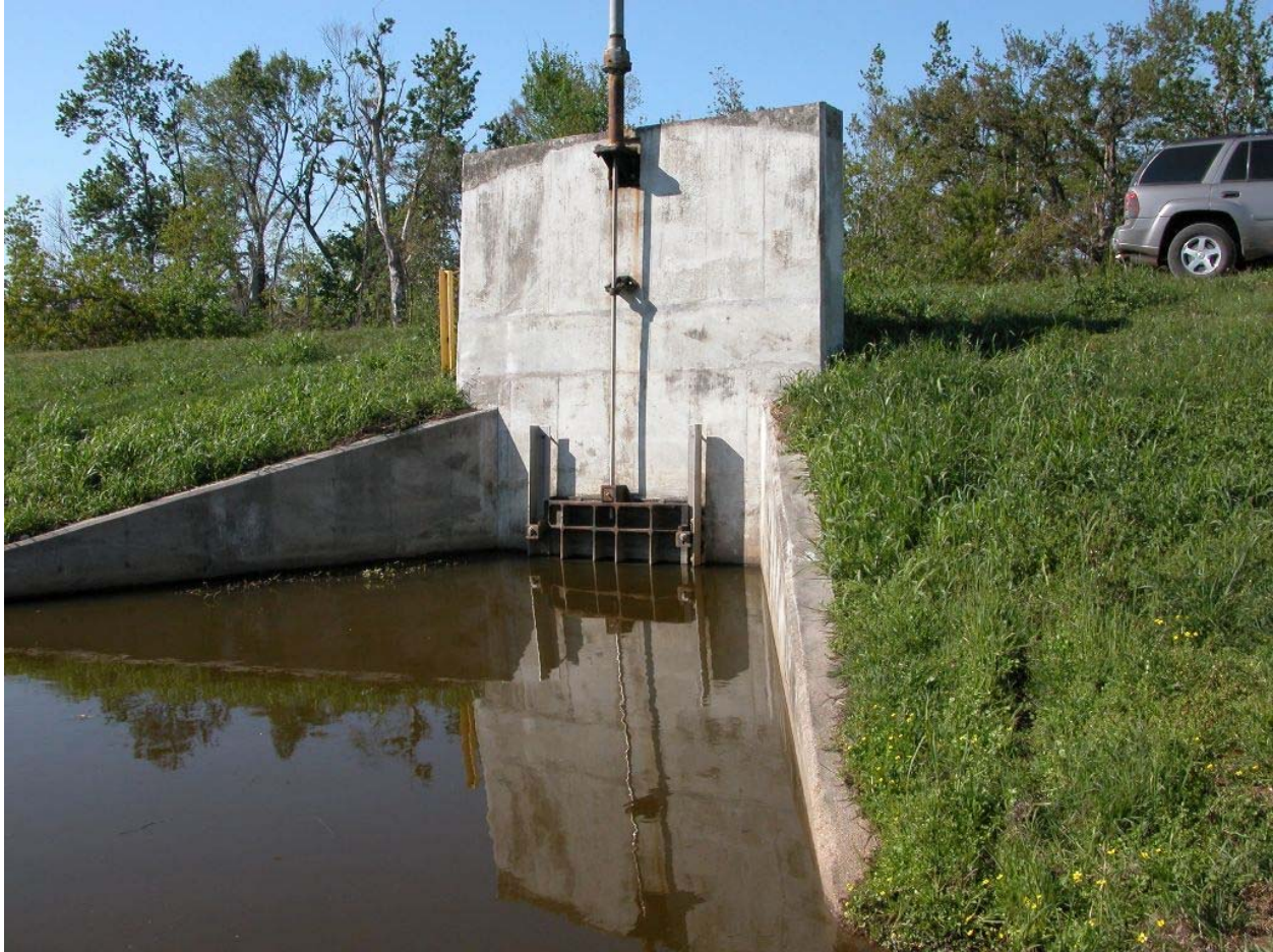
Drainage structure under Back Levee outside U.S. Coast Guard station. Screw gate closure on culvert
