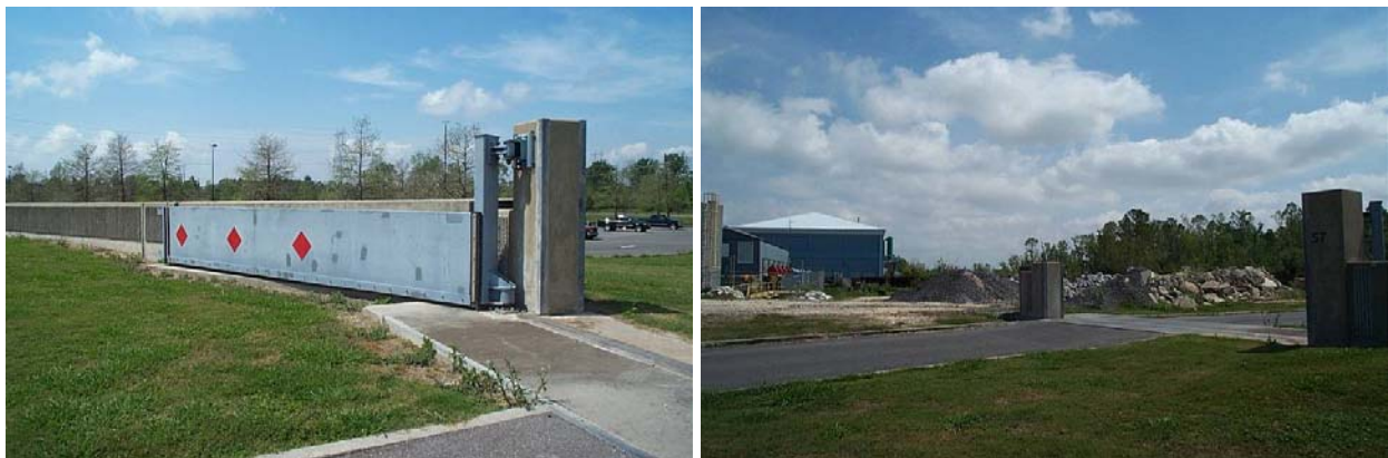
Swing in the concrete capped I-wall at the Segnette State Park where wall ends at the Segnette Pump Station
