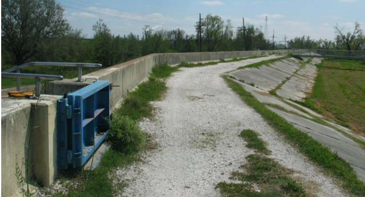
Figure STB 20. Concrete capped I-wall along Miss. River near Battlefield (access closure gate is key point within this reach)
