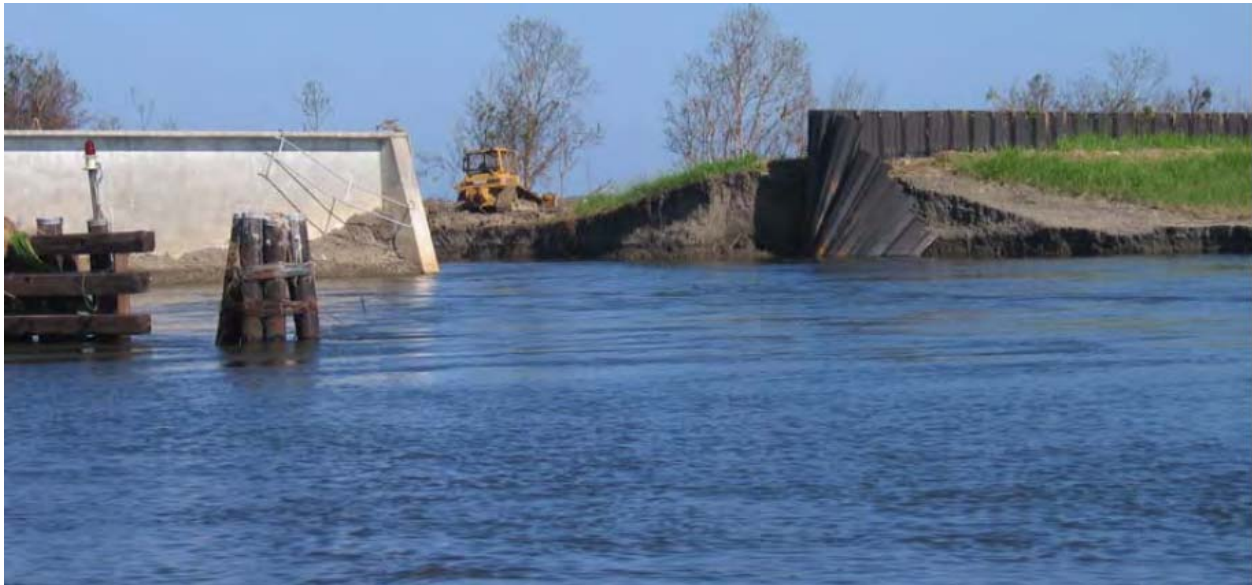
Figure STB 14. Picture of breached Bienvenue I-wall from Protected Side
