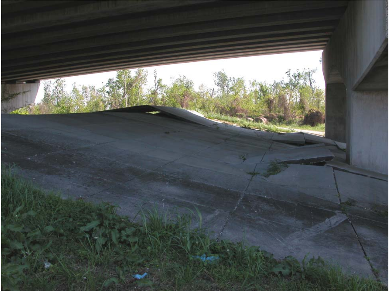
Back Levee passed under General De Gaulle onramp from Hwy 406. Buckling of concrete slab on levee under ramp.
