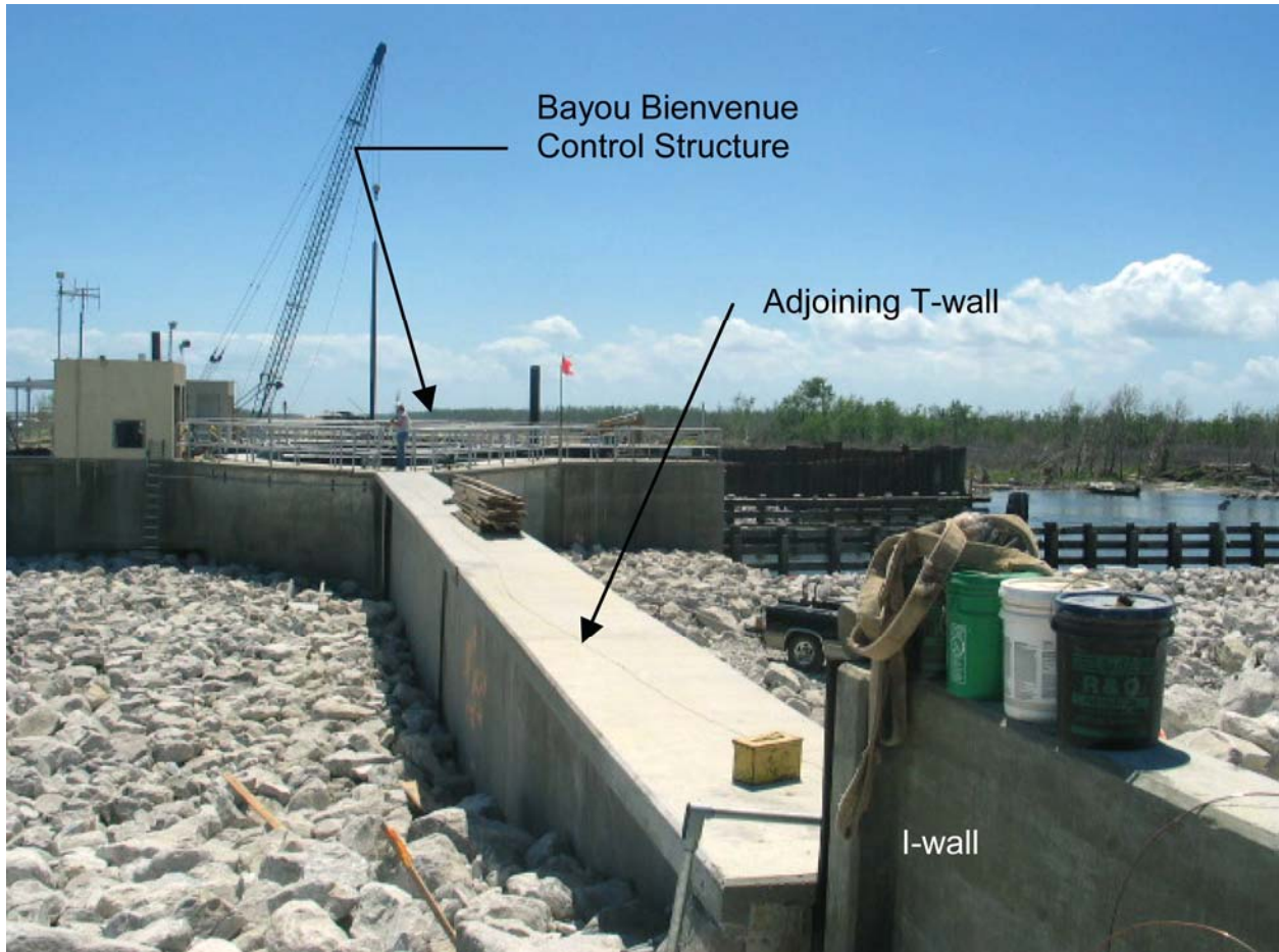
Figure STB 34. Riprap placement around Northwest Floodwall adjoining Bayou Bienvenue Control Structure (looking southeast along MRGO)
