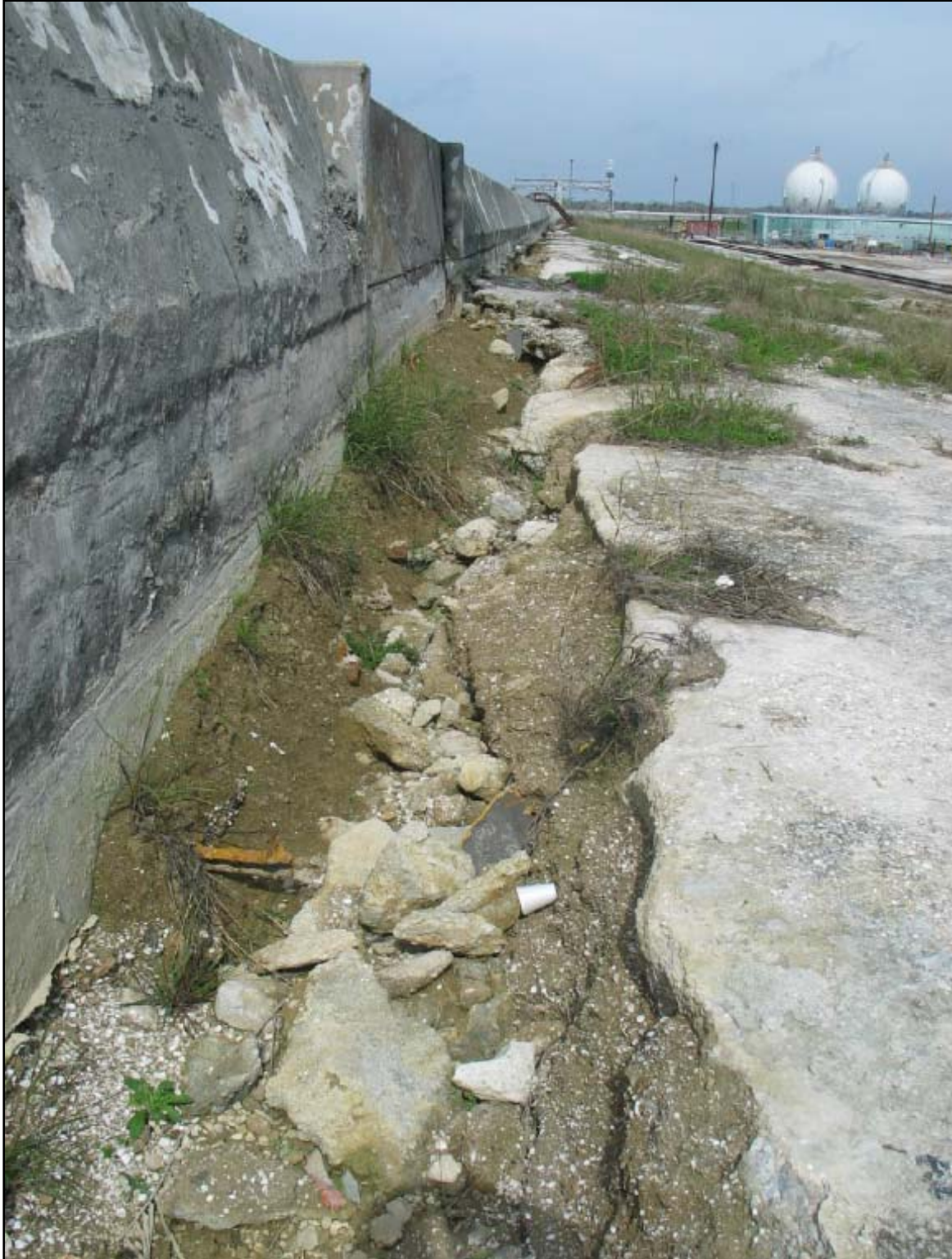
Figure NOE 14. Scour Damage Behind Michoud Canal Floodwall
