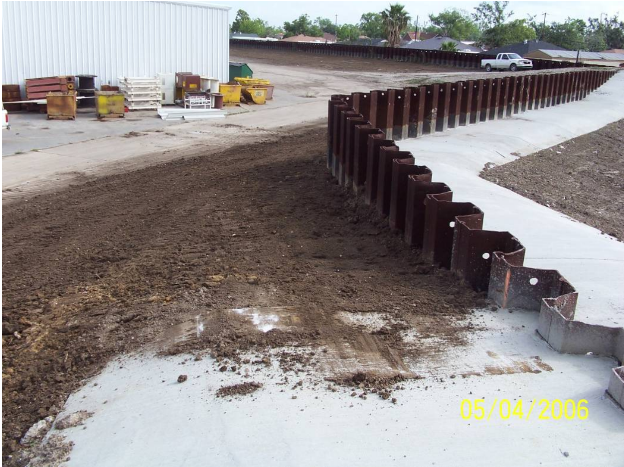
Figure STB 38. Scour repairs to Caernarvon sheetpile I-wall area (Note: compare to pre-Katrina condition shown in Figure STB 18)
