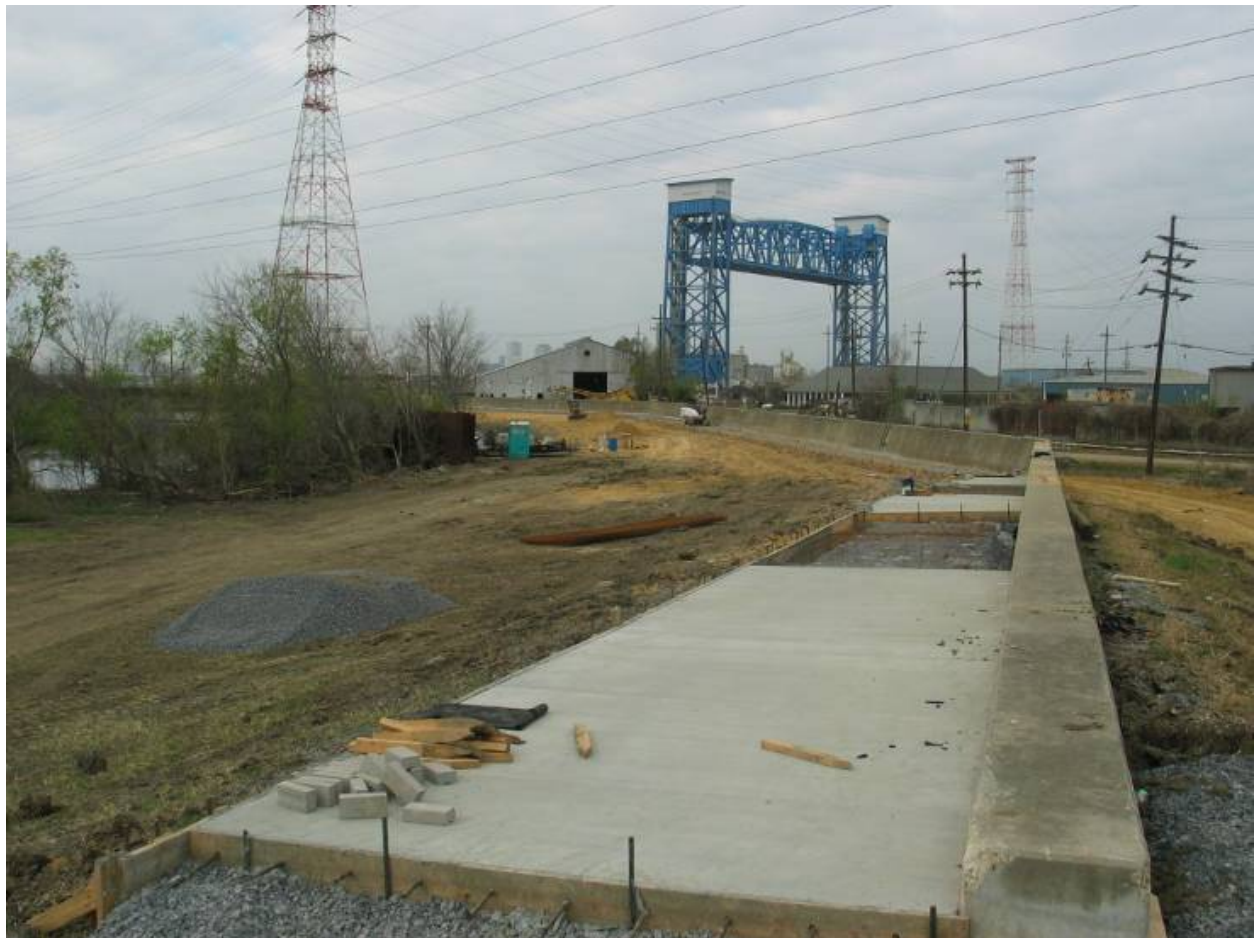
Figure STB 30. New scour protection pad (typical) (photo taken at end of Reach STB4 looking back toward IHNC)
