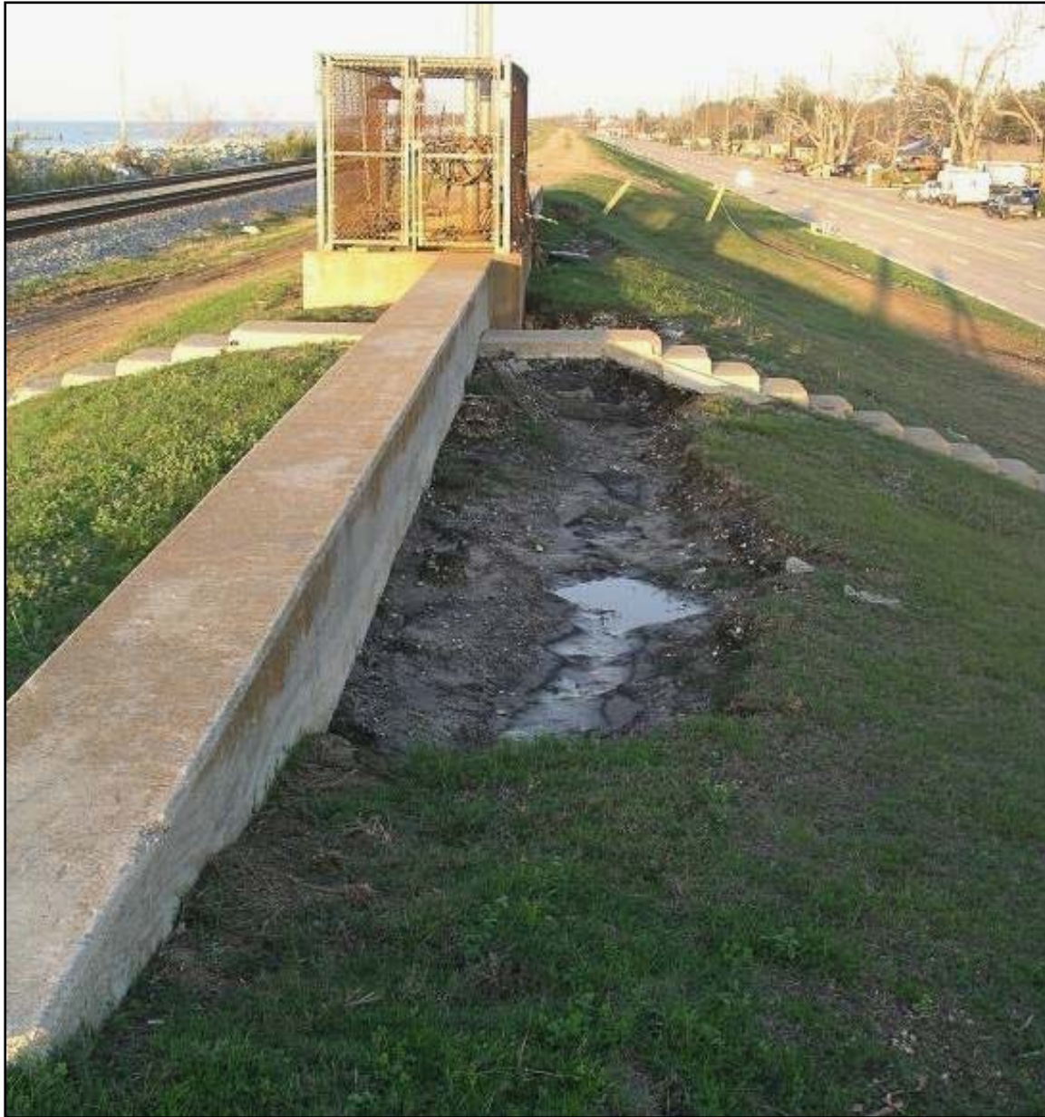
Figure NOE 7. Minor Scour from Overtopping at Jahncke Pump Station
