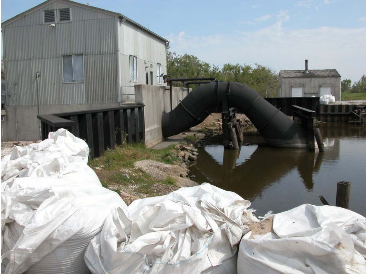
Ollie Pump Station
