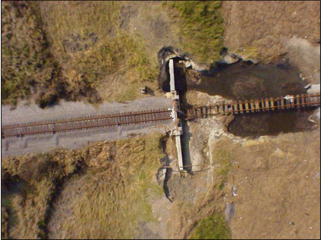
Figure NOE 10. Aerial View of Damage at RR Closure Along East Levee
