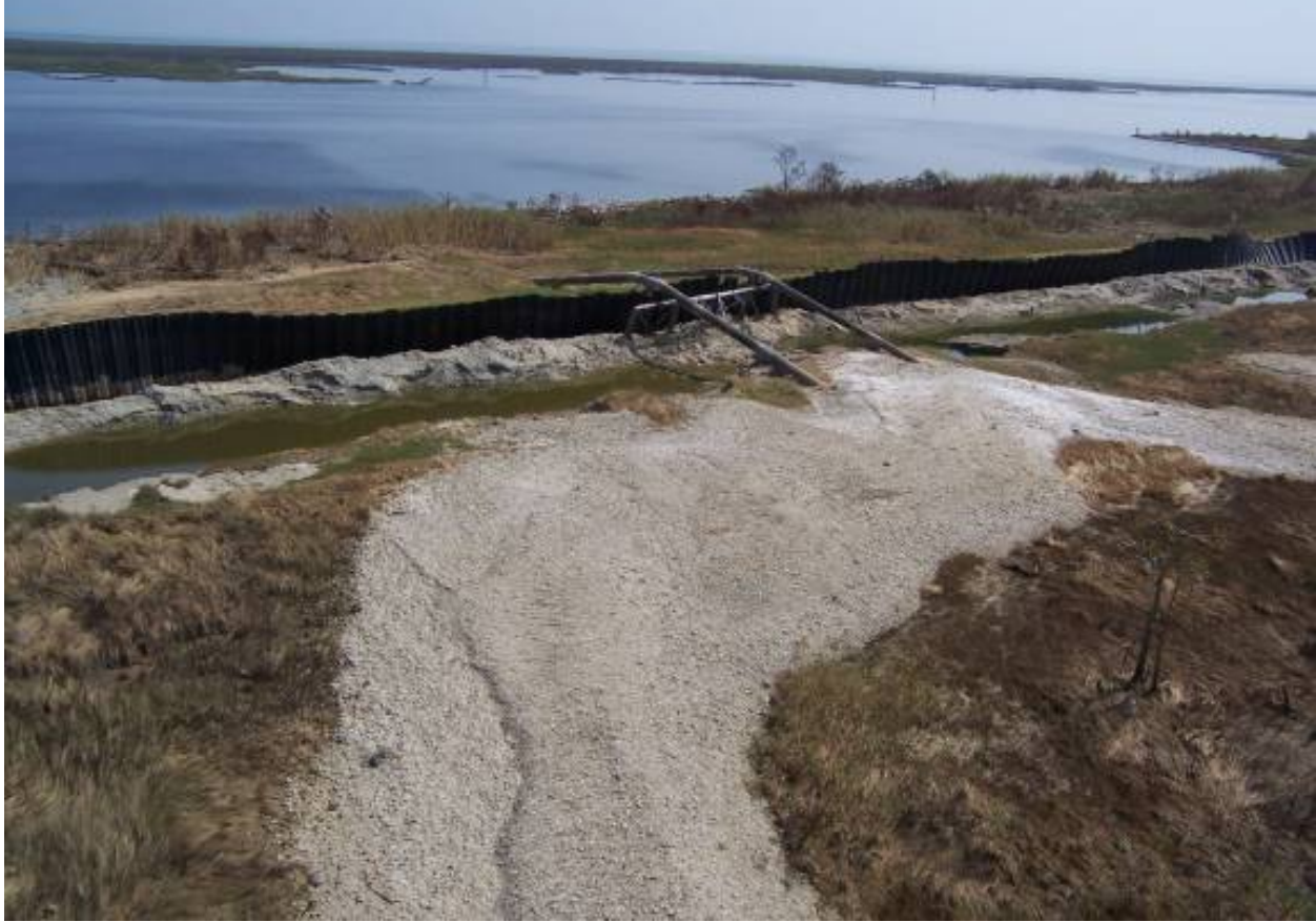
Figure STB 15. Breached I-wall along MRGO
