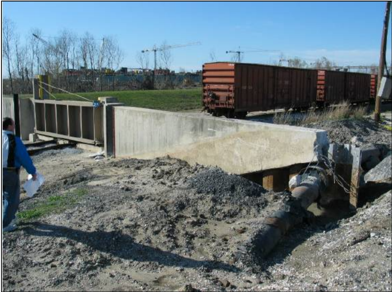
Figure NOE 17. Erosion Damage Around RR Closure (Near GIWW and IHNC Intersection)
