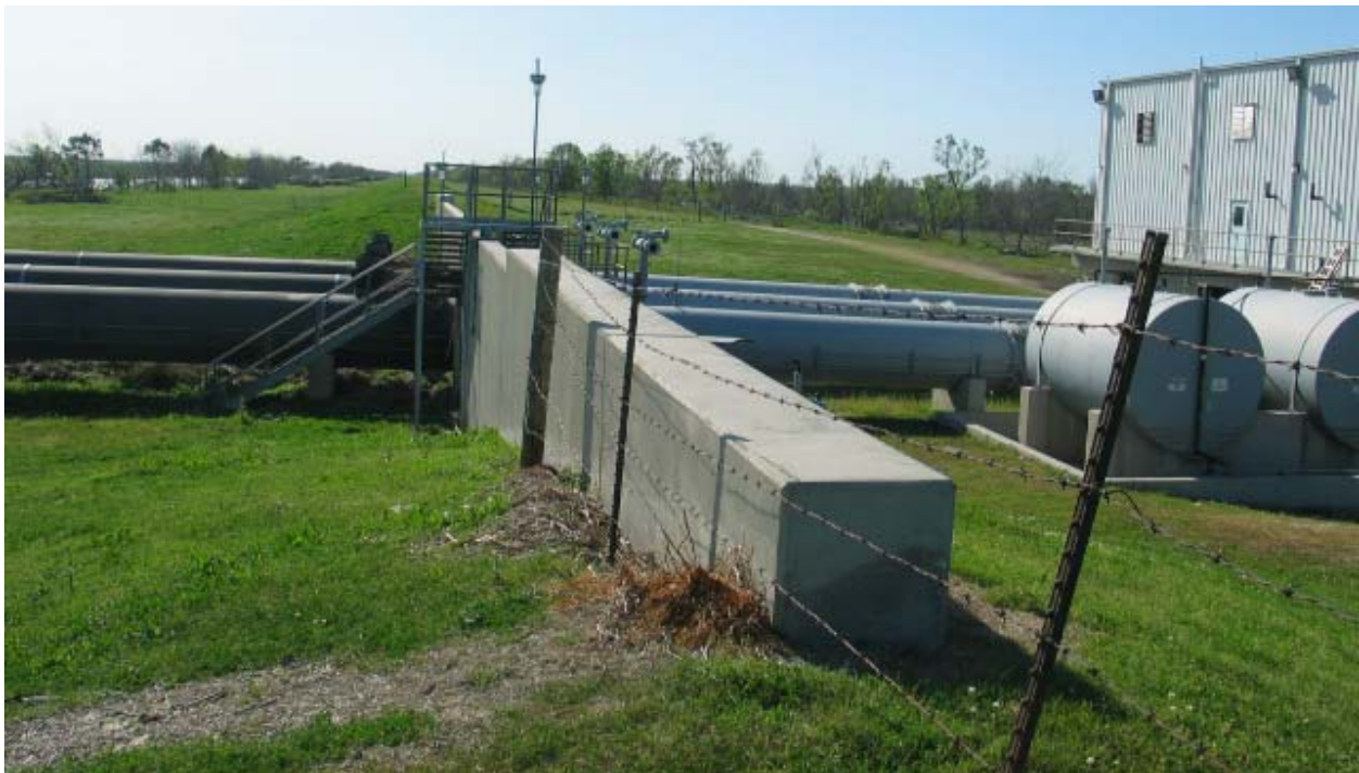
Figure STB 17. Floodwalls surrounding Pump Station #8 pipes (viewed Looking West Along Caernarvon Canal)
