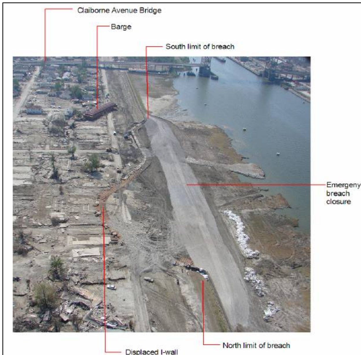
Figure STB 5. Failed I-wall section of Lower 9th Ward (Reach STB2) (looking south along IHNC)
