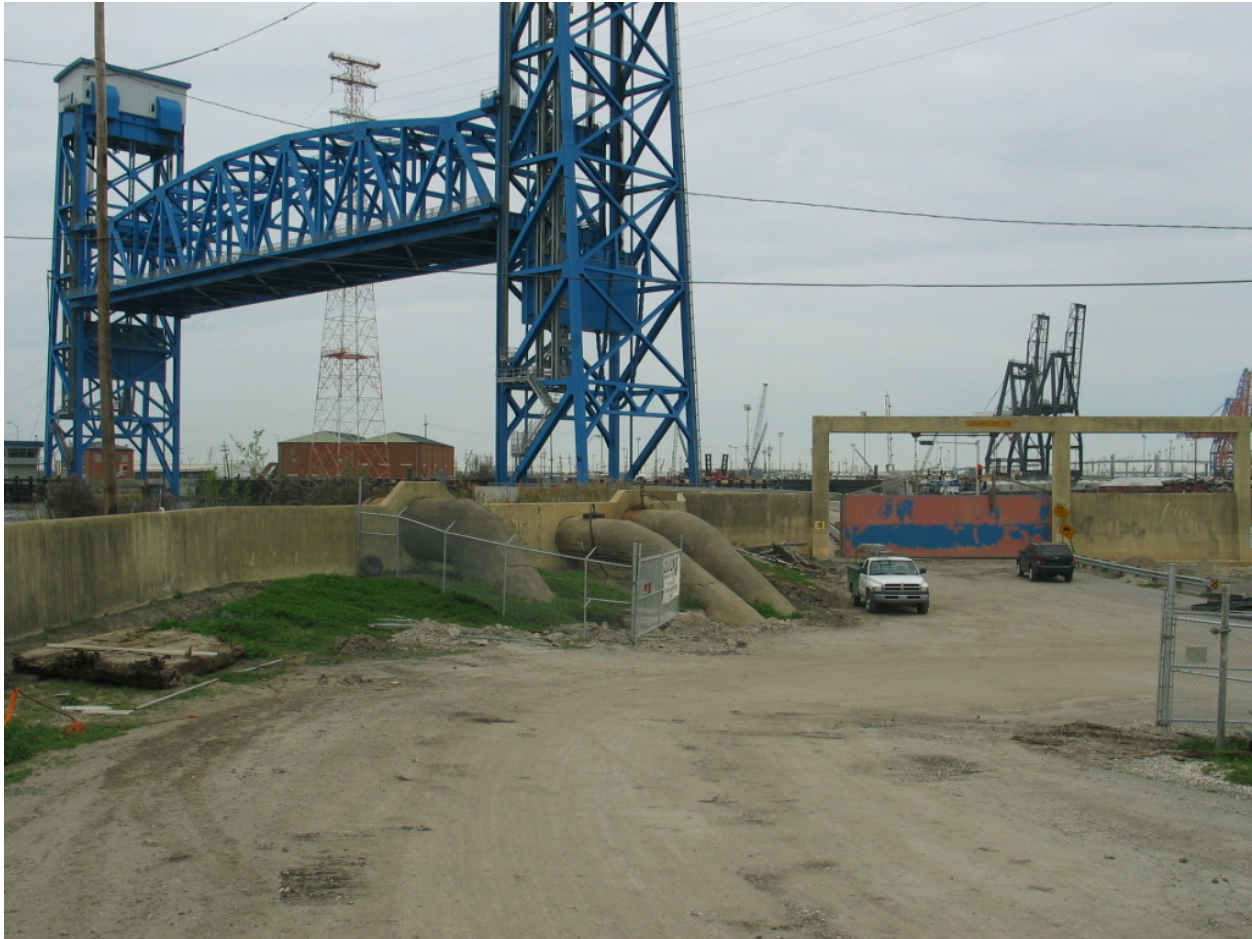
Figure STB 8. Existing T-wall near Florida Ave. Bridge (Reach STB3) (looking from protected side towards IHNC)
