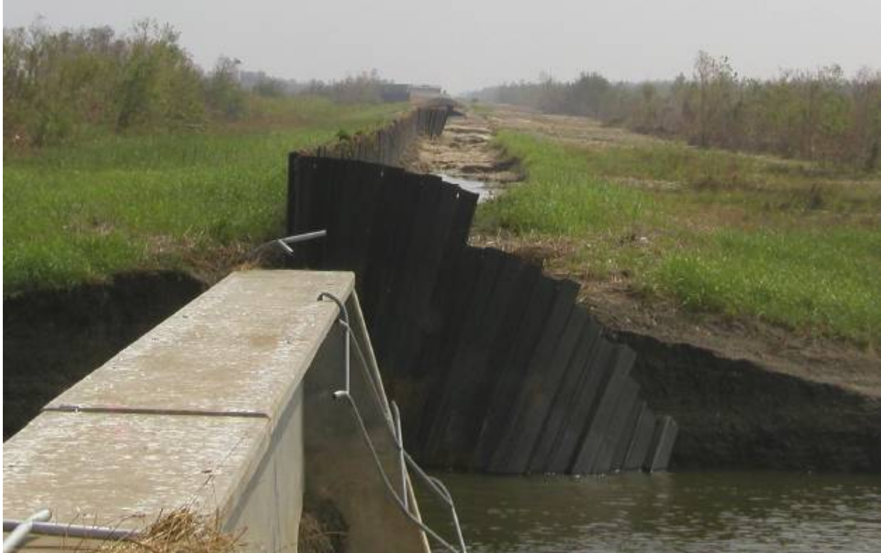
Figure STB 13. Uncapped I-wall Section on Southeast side of Bayou Bienvenue Control Structure (looking southeast along the MRGO)
