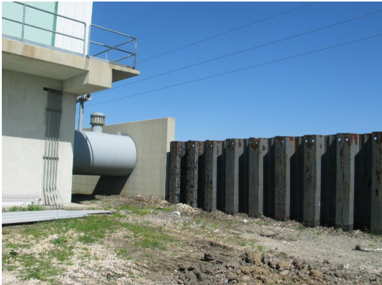
Figure STB 26. T-wall and I-wall offset at Pump Station #7 along interior local levee (Note: wall offset is approximately 3.5 feet)
