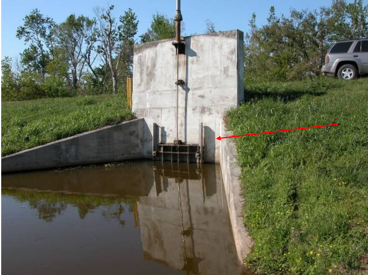
Drainage structure under Back Levee outside US Coast Guard station. Screw gate closure on culvert
