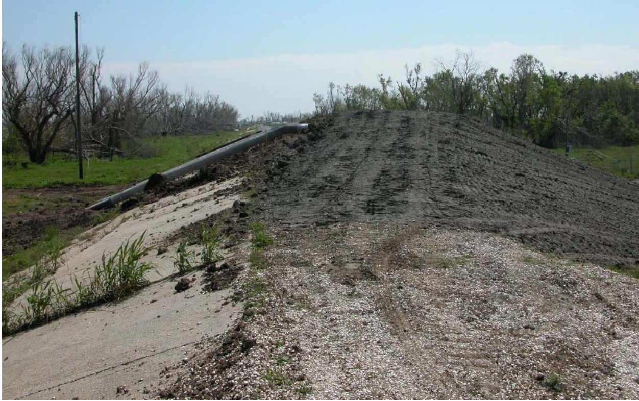
There were a few cases of erosion along the MRL
