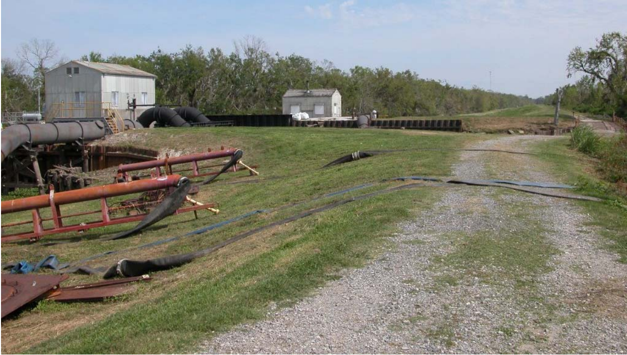
Ollie Pump Station
