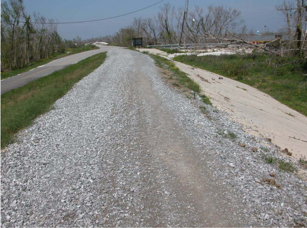
More typical condition along this section of the MRL, with concrete paved or stone crown and concrete armored floodside
