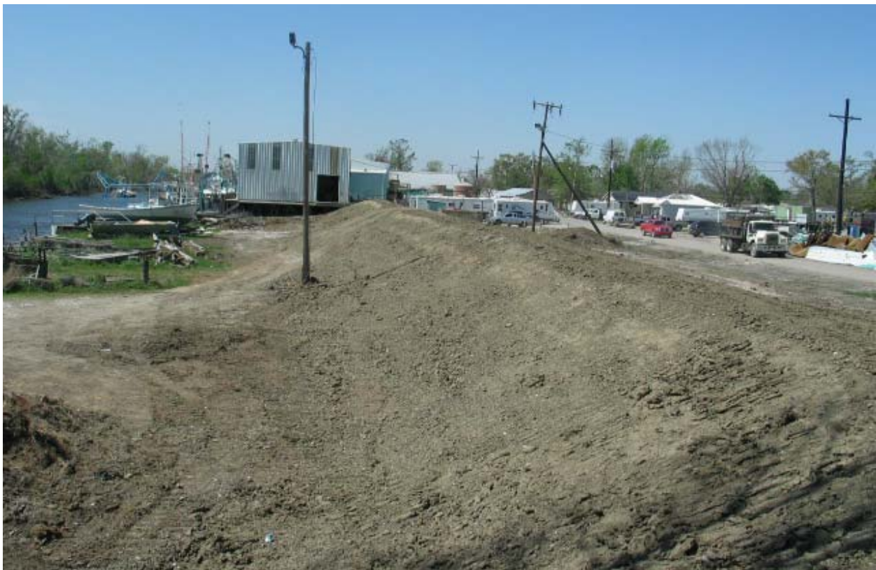
Figure STB 40. Repairs and levee raising to Reach STB39 along Violet Canal (viewed looking west from end of Reach STB38)
