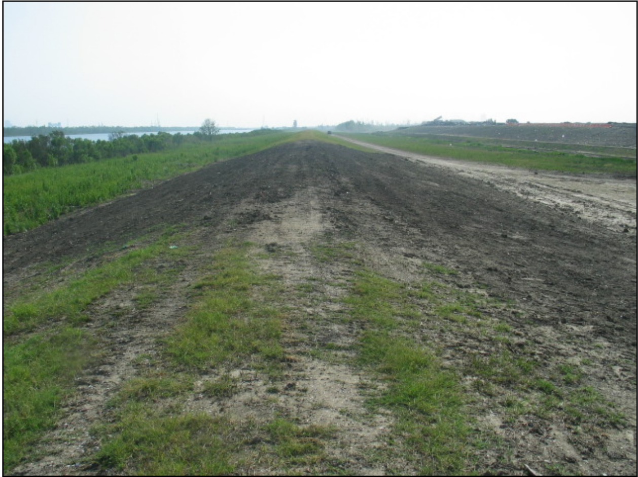
Figure NOE 33. Scour Damage Repairs Along Citrus Back Levee (Note: reference Figure NOE 15 which shows damage following Katrina)
