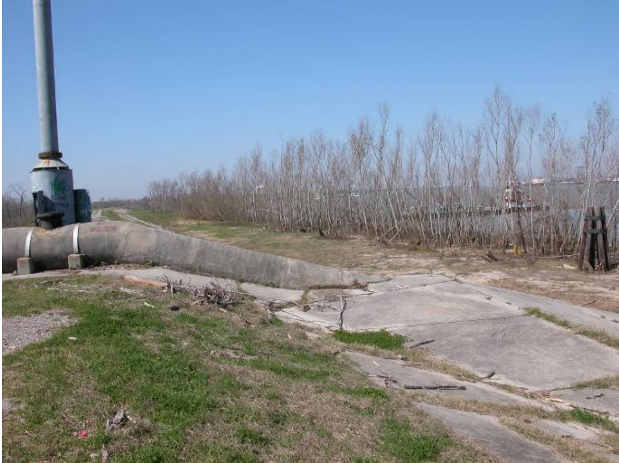
Pipe crossing along MRL just east of GIWW and MRL intersection
