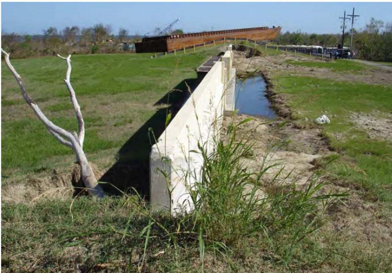
Figure STB 11. Floodwall Northwest of the Bienvenue Structure (Reach STB10) (looking southeast toward Bayou Bienvenue just after Katrina)
