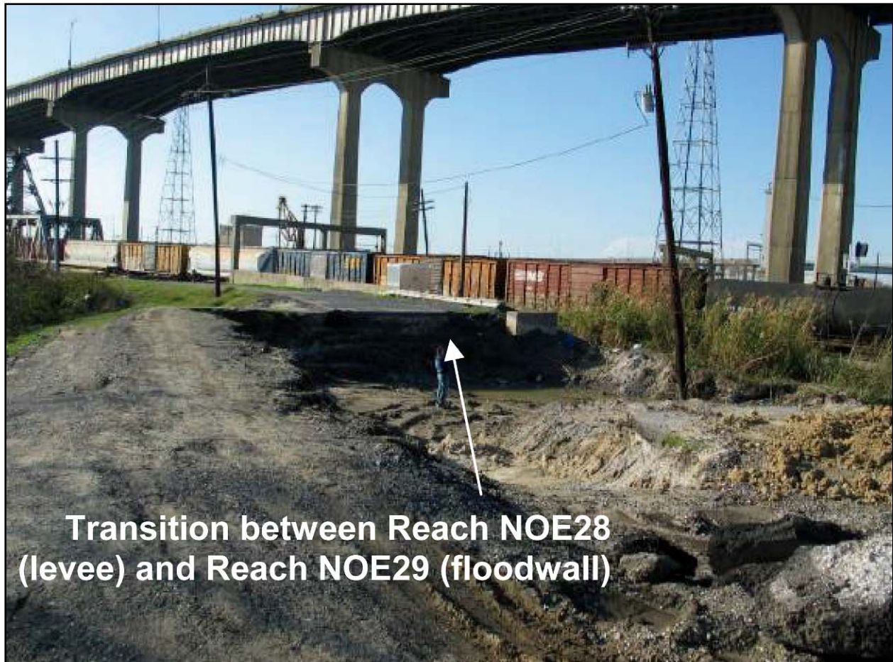
Figure NOE 19. Major Washout Area from Overtopping Near I-10 Overpass (Note: Located Along IHNC East Side)
