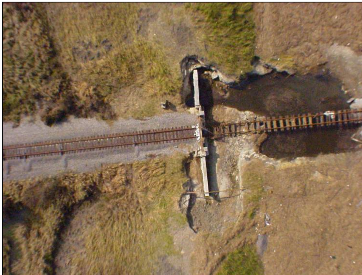
Figure NOE 10. Aerial View of Damage at RR Closure Along East Levee
