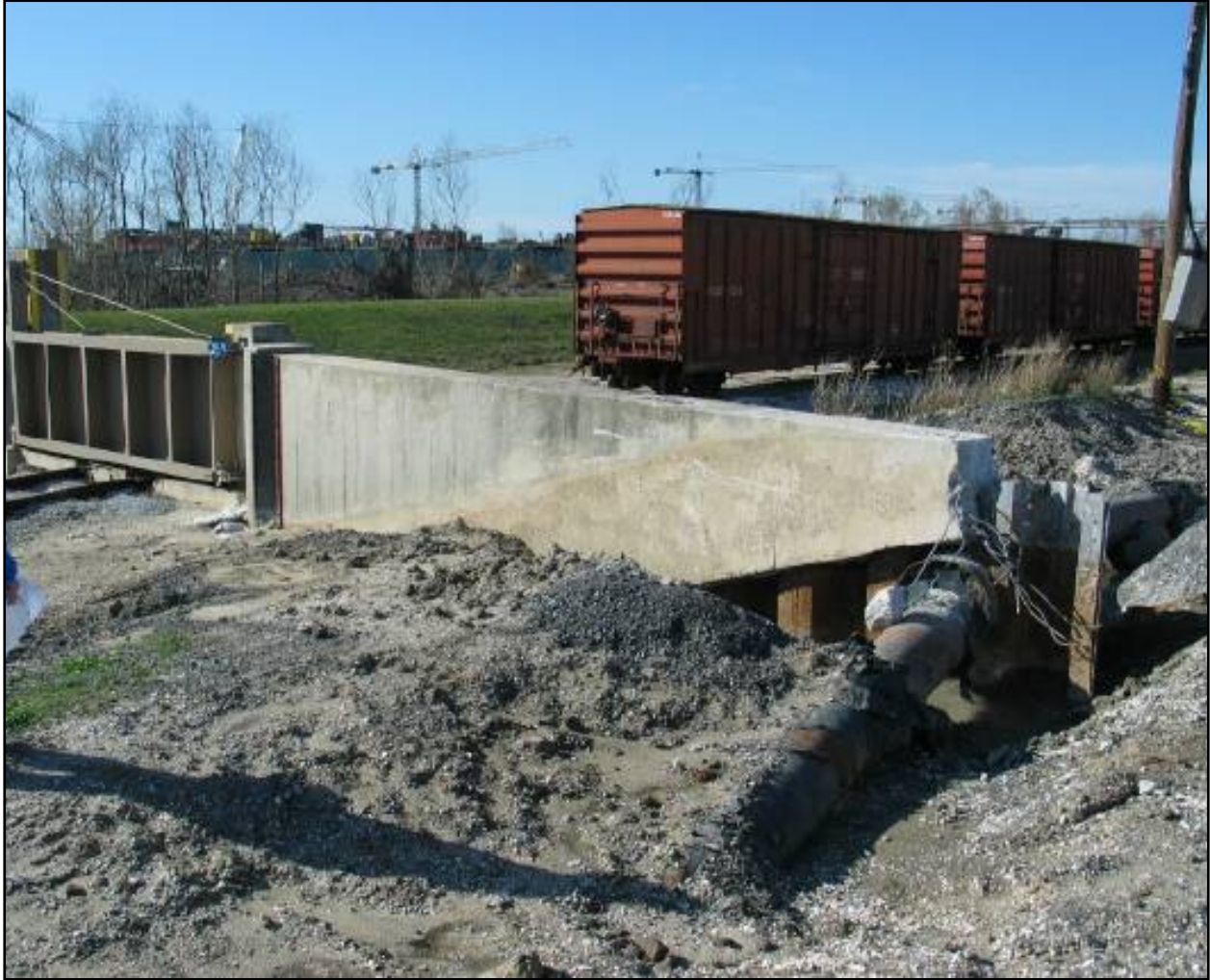
Figure NOE 17. Erosion Damage Around RR Closure (Near GIWW and IHNC Intersection)
