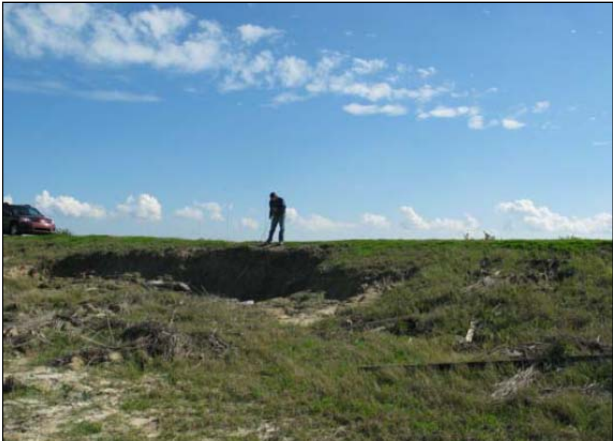
Figure NOE 15. Scour Damage Along Citrus Back Levee
