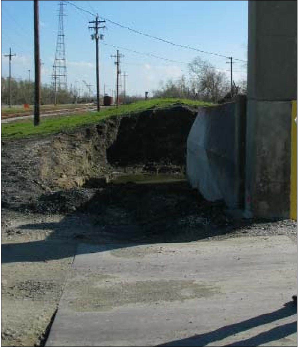
Figure NOE 18. Scour Damage around Gated Closure Along IHNC
